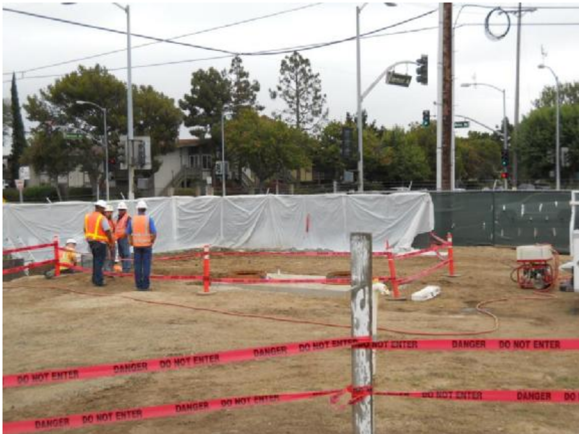
Figure 13: General site view of Injection Well 5
