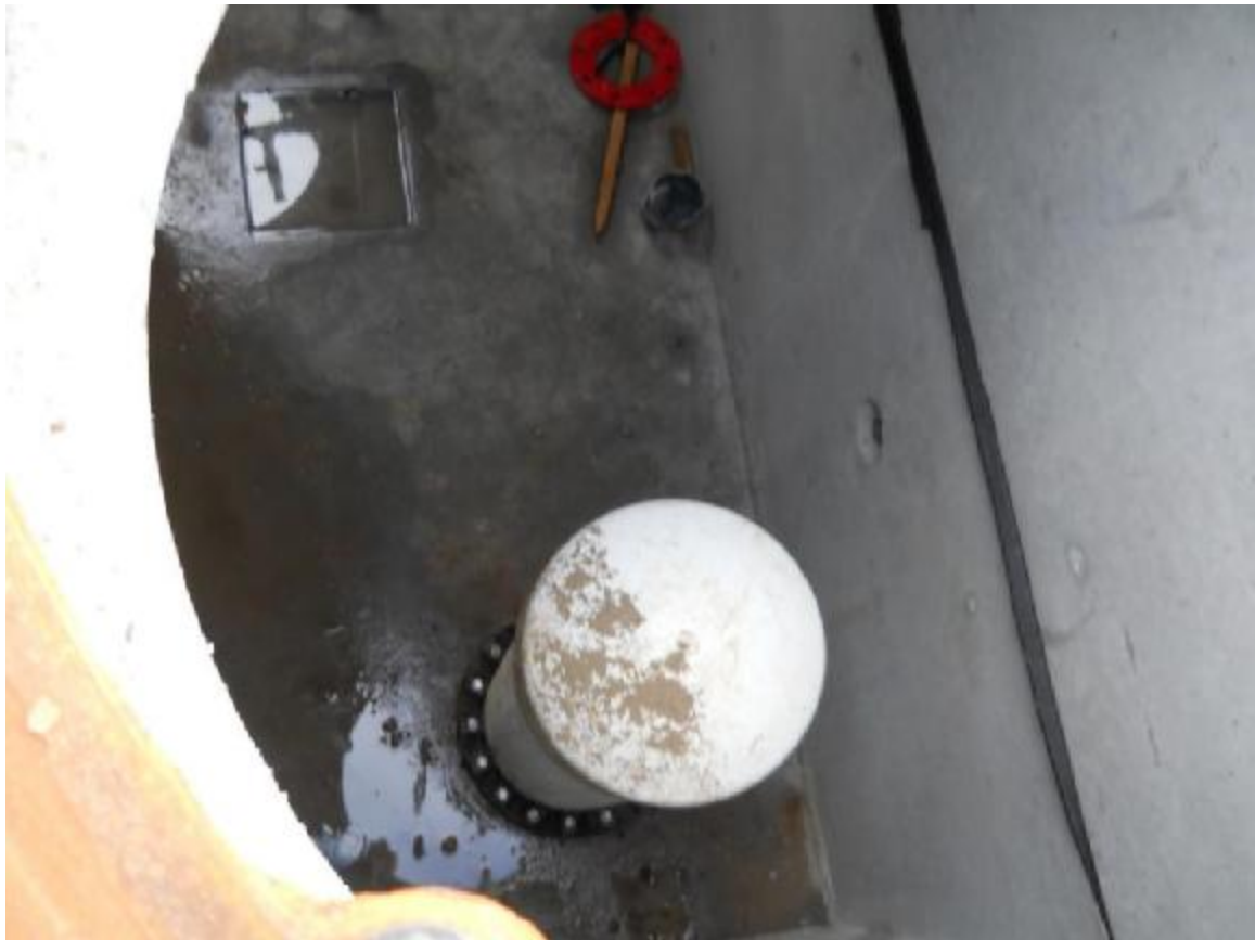
Figure 5: Inside IW5 with pressure gauges
