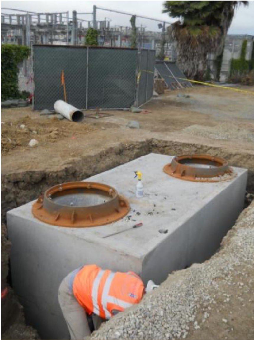
Figure 2: Injection Well 2 (IW2)
