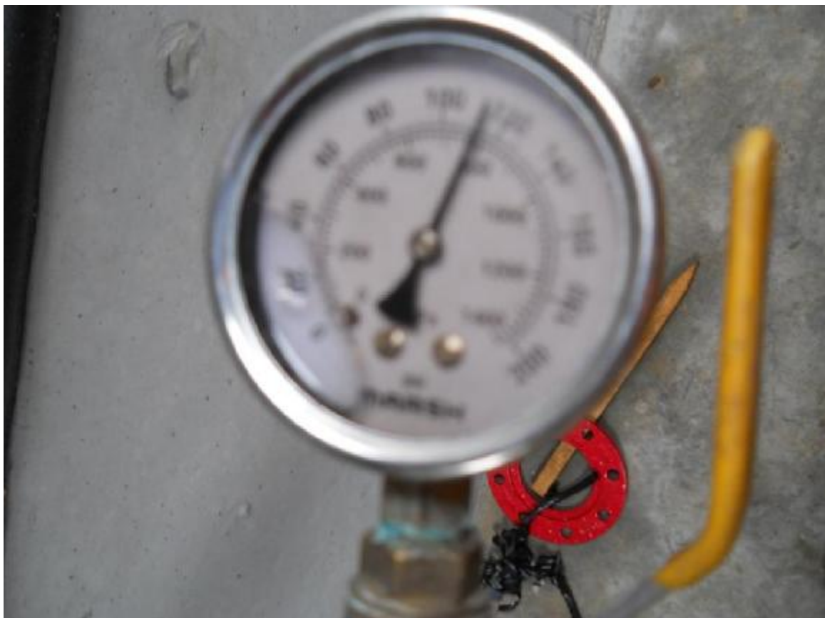
Figure 10: Close-up view of pressure gauge on 4-inch redevelopment return line
