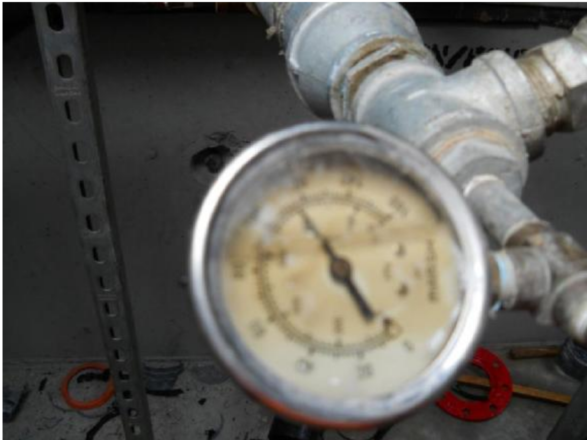
Figure 9: Close-up view of pressure gauge for 4" injection line with 6" header
