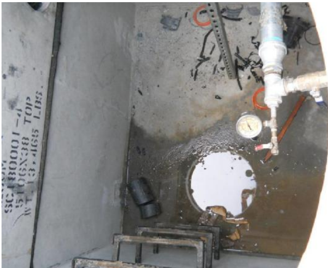
Figures 6: Pressure gauge for 4-inch Injection line with 6-inch header
