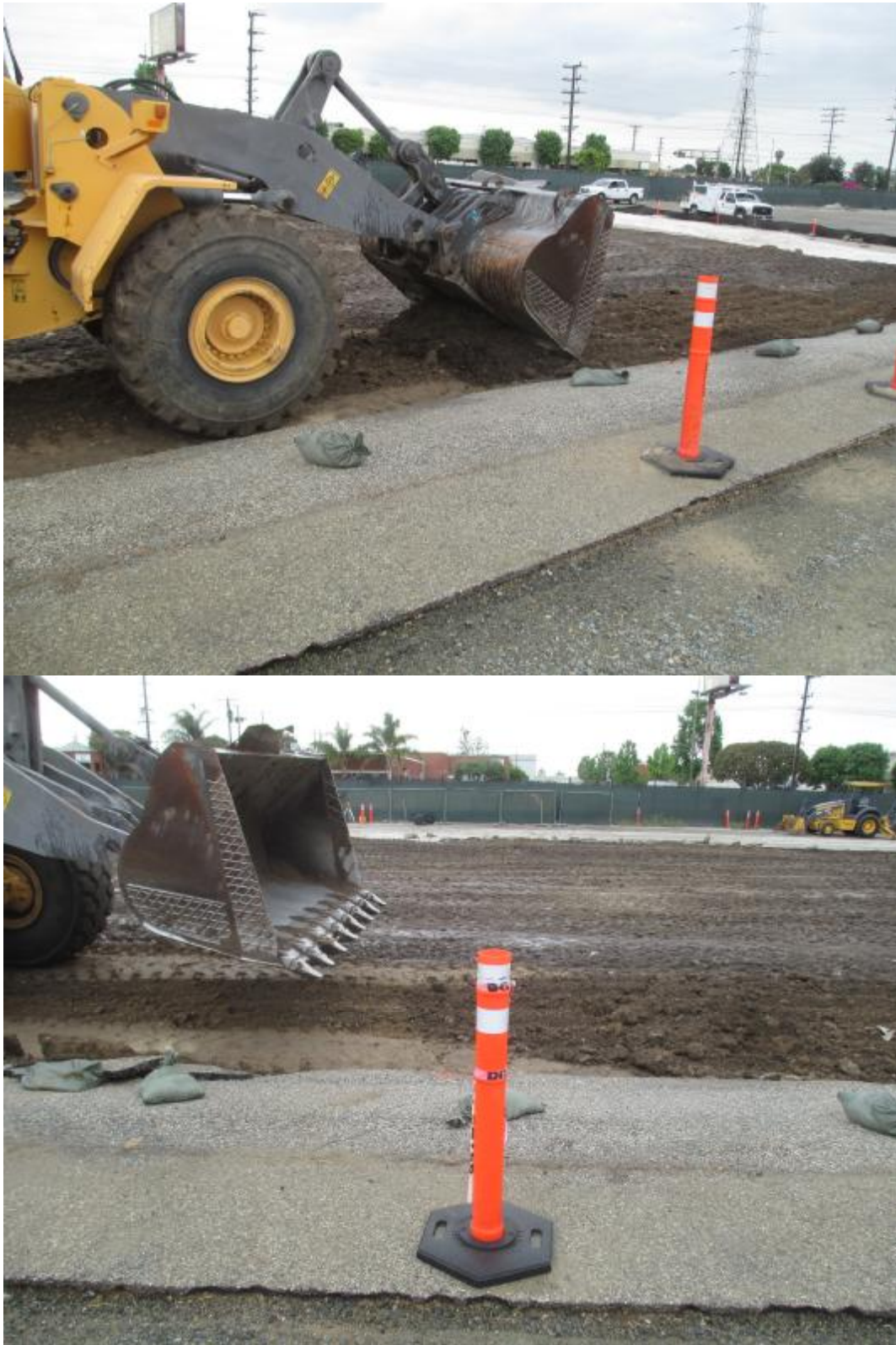
Figure 2: Blended soil being placed in thin layers and back dragged by loader.
