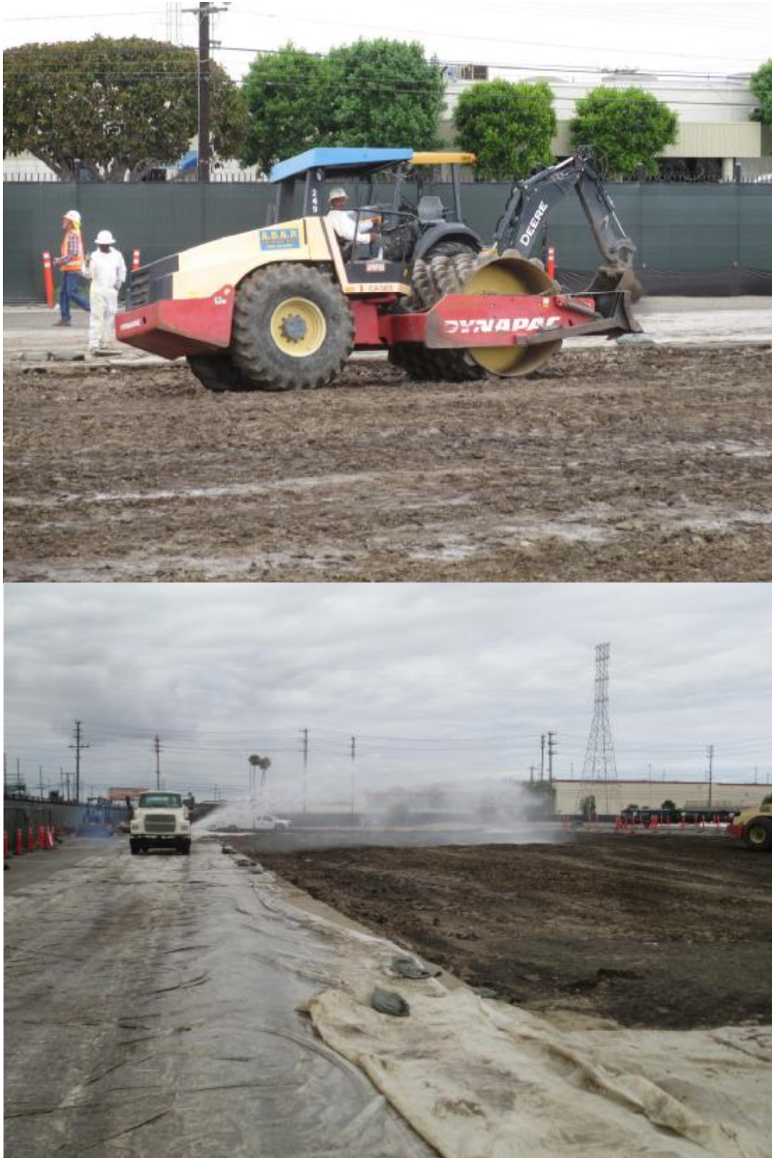
Figure 3: Sheep's foot dynamic compactor working fill (top) and water truck spraying fill (bottom).
