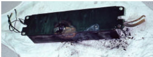
This ballast sparked a fire at a school in Southern California in 1999.
