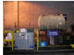
PCB Processing Area
