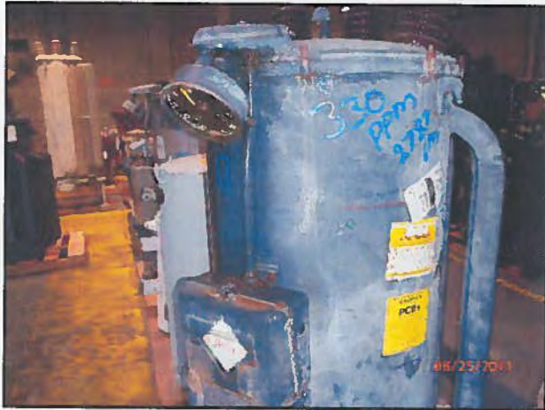
Photo 4 – Transformer Marked as "330 ppm"
