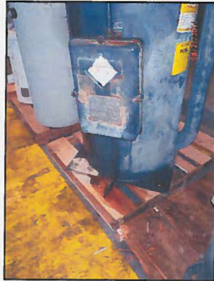
Photo 5 – Liquid on Floor & Pallet
