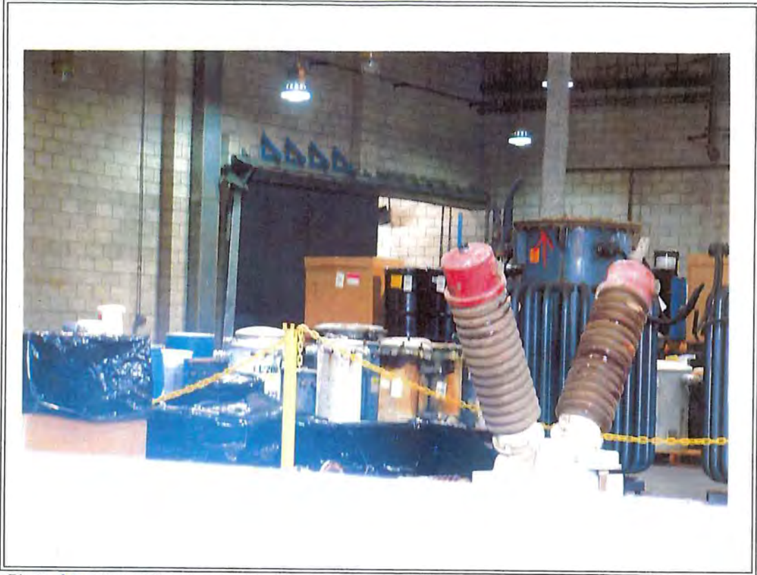
Photo 12 : View of Bushings & Transformers inside CHI "Container Storage Warehouse."
