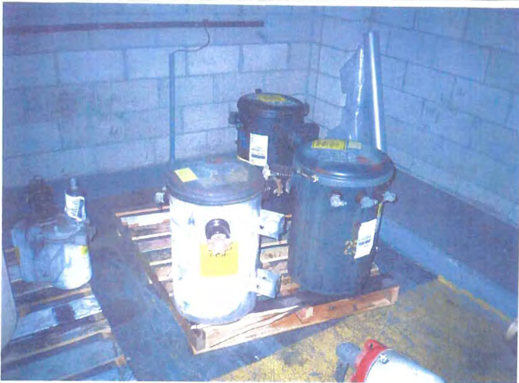
Photo 15 : View of PCB transformers inside CHI "Container Storage Warehouse."
