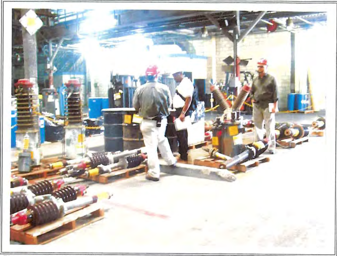
Photo 10 : View of more bushings & transformers inside CHI "Container Storage Warehouse" w/ Chris, Roger Fox, & Brian Olson.
