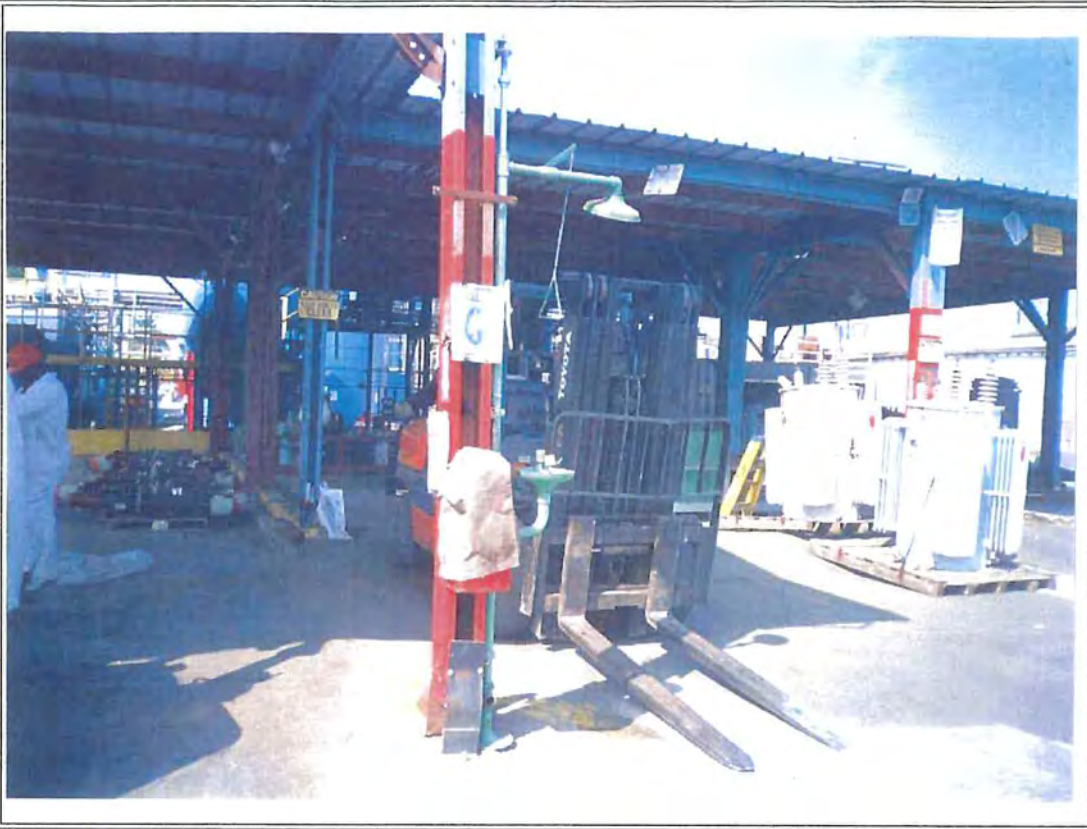
Photo 6 : Closeup of tanker unloading facility showing transformers awaiting processing.
