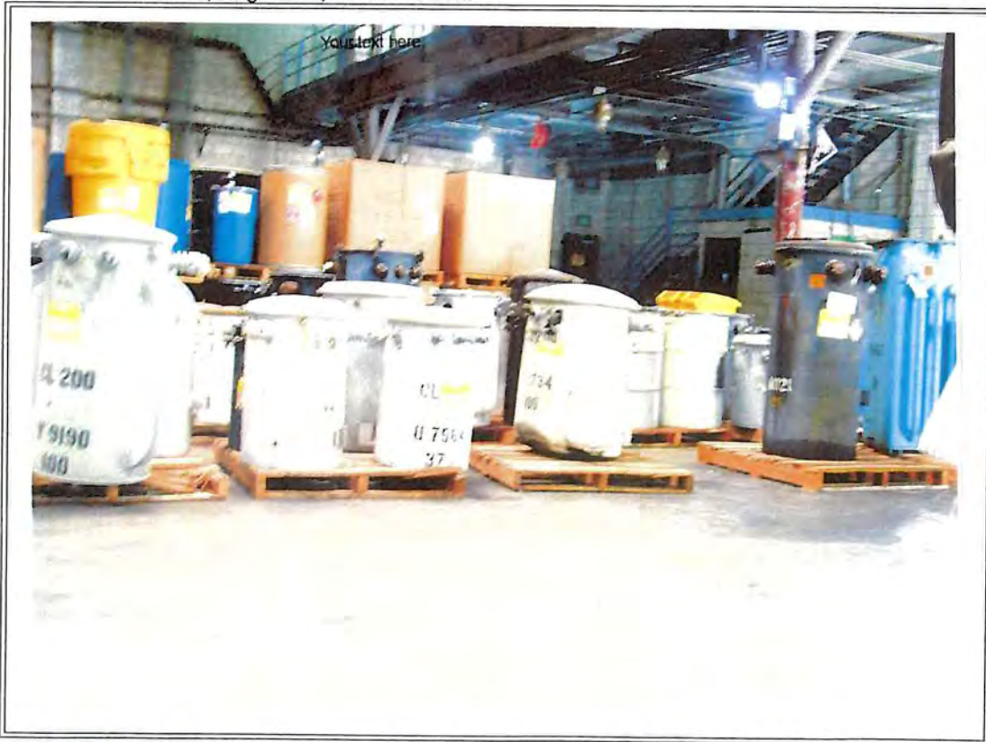
Photo 11 : View of transformers stored inside CHI "Container Storage Warehouse."
