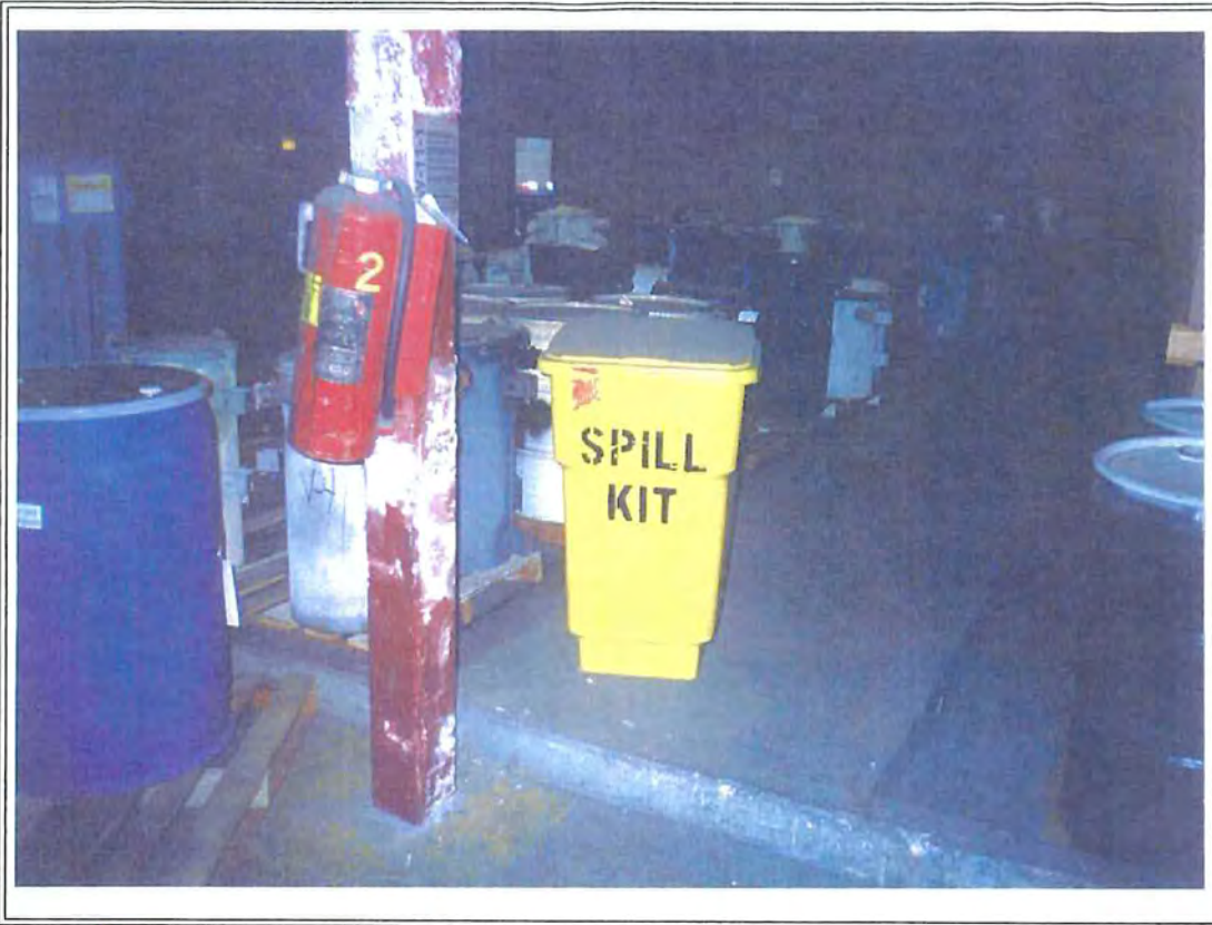
Photo 14 :View of emergency spill kit inside Container Storage Warehouse.
