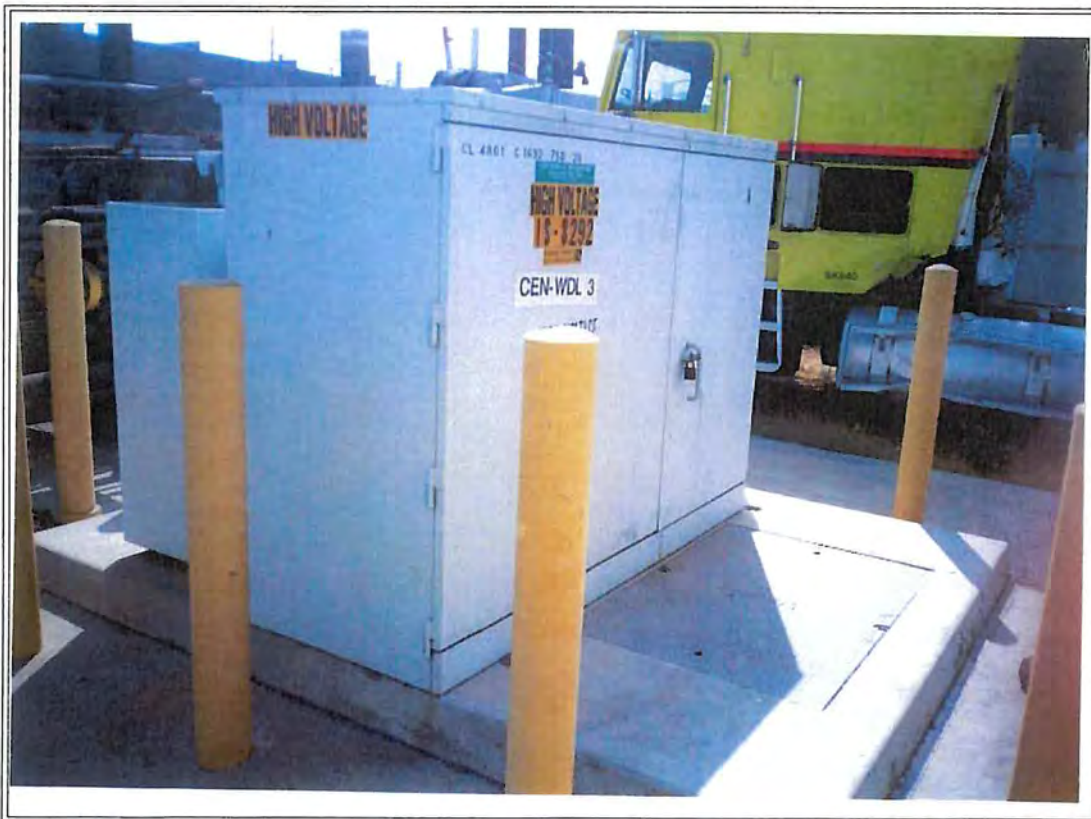
Photo 7 : View of pad transformer supplying power to transformer processing facility.
