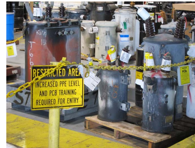
PCB Equipment in Storage
