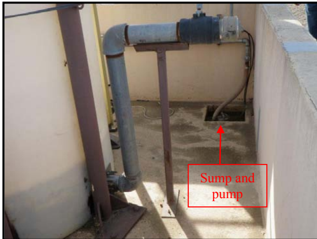
P-9: Pump-out connection used to remove the contents from the 90-day hazardous waste storage tank. Note: The sump has a pump which is used to transfer any fluid which may accumulate from rainfall events into the P-9 leachate collection tank.
