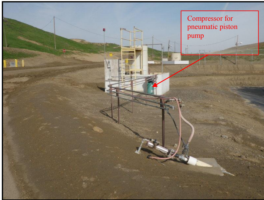
P-9: Riser assembly in the foreground leading to the leachate collection tank (facing north). A pneumatic piston pump is used to pump out the leachate sump.
