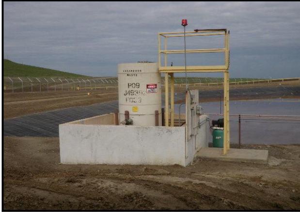
P-9: Leachate Collection Tank (facing east). Note: The panel on the right side contains the high level alarm and the magnehelic device used for determining the sump liquid level.
