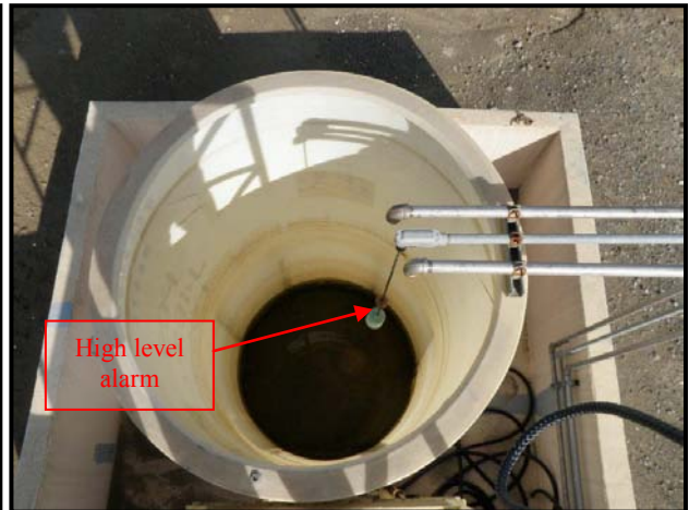
The leachate collection tank at P-9 is an open-top tank. Three pipes are located on top of the tank. One pipe is from the P-9 riser assembly, one pipe is from the P-9 tank sump, and the middle pipe is the high level alarm which ensures that the two-foot freeboard is maintained. The inspectors observed several inches of rainwater on the bottom of the tank, as described on the label.
