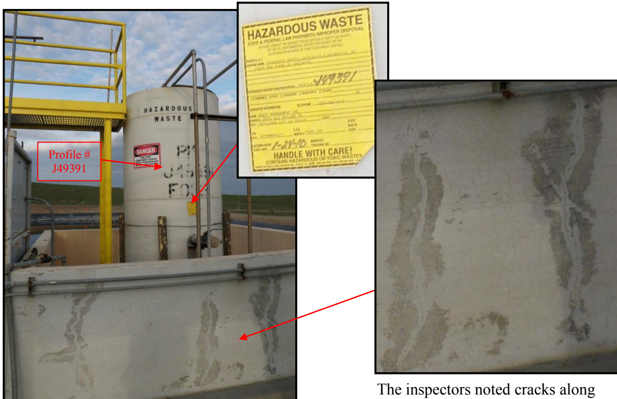
P-16: Leachate Collection Tank (facing east). Note: The panel on the left side contains the high level alarm and the magnehelic device used for determining the sump liquid level. The inset HW label is cropped and enlarged.
