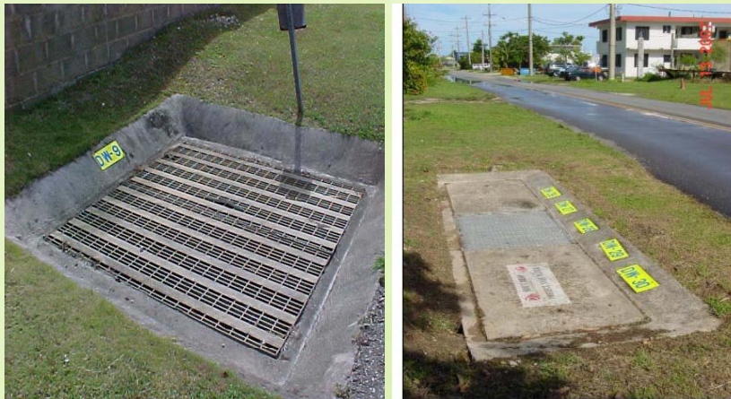
Bored or Drilled UIC Wells in Concrete Vault
