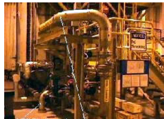
LFG-fired Boiler Ft. Wayne, IN
