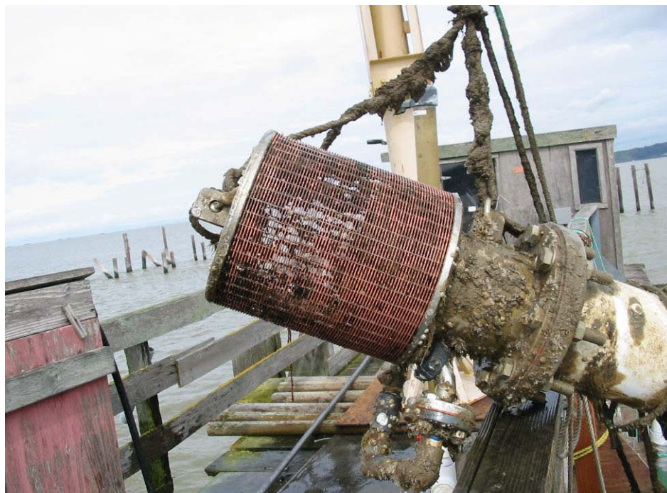
Figure 8-5: Marin Municipal Water District (MMWD) Seawater Desalination Pilot Program Intake Screen after Manual Cleaning
