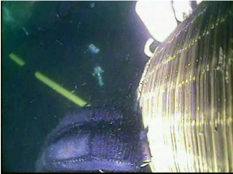
Figure 9-3: Pilot Intake Screen Mounted in the Water off Santa Cruz Wharf (Tenera, 2010)
