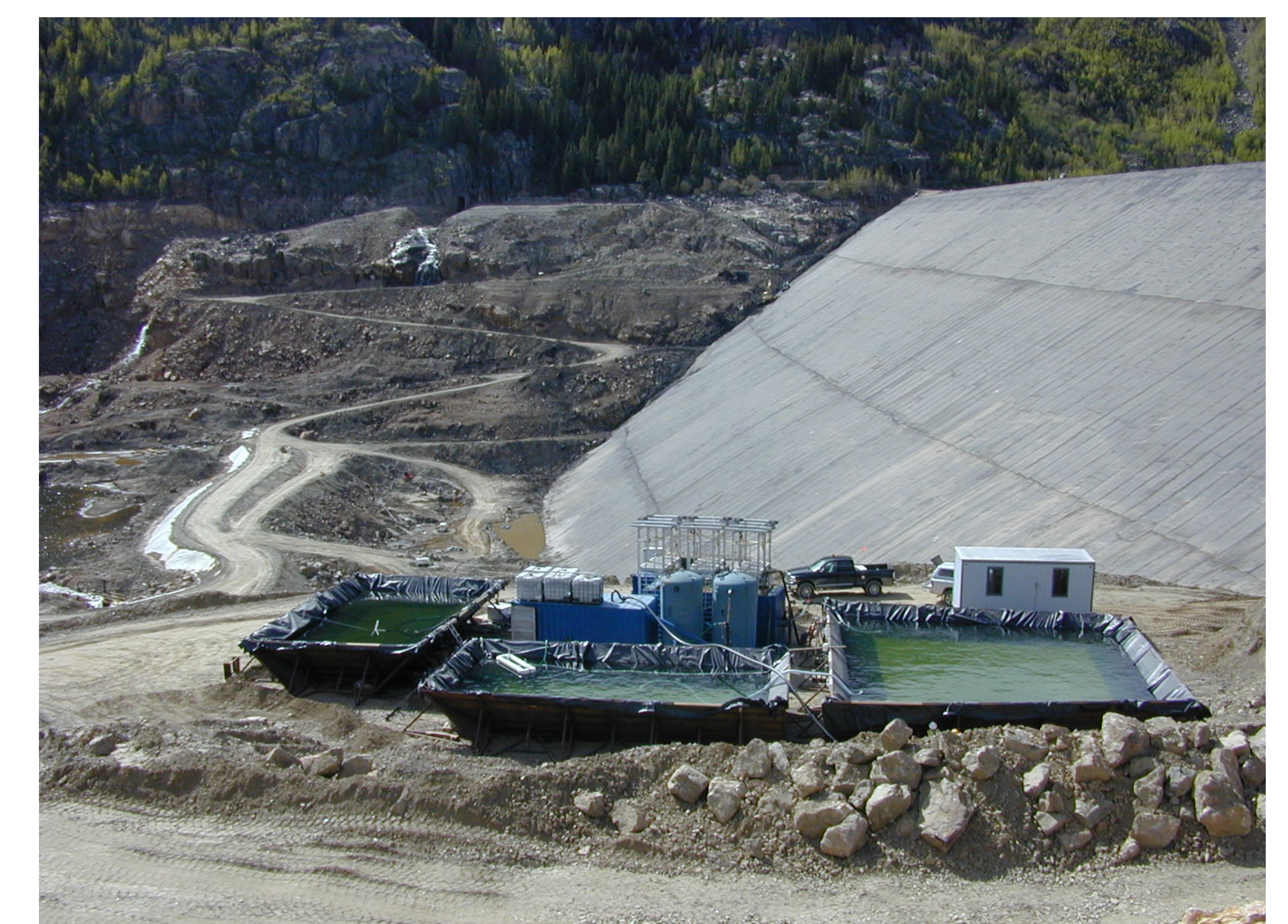
Figure 3: The EC system was set up to treat water that had been used in the resurfacing of a dam. The water was recycled for reuse.
