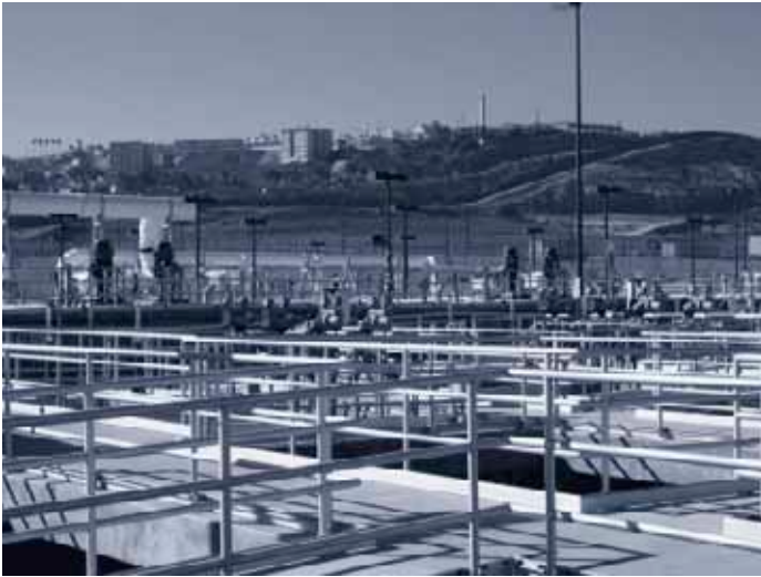
The South Bay Water Reclamation Plant has the capacity to treat 15 MGD of wastewater from the South Bay District of San Diego County to meet tertiary treatment standards. Reuse of treated wastewater can help relieve the heavy demand on limited resources.
