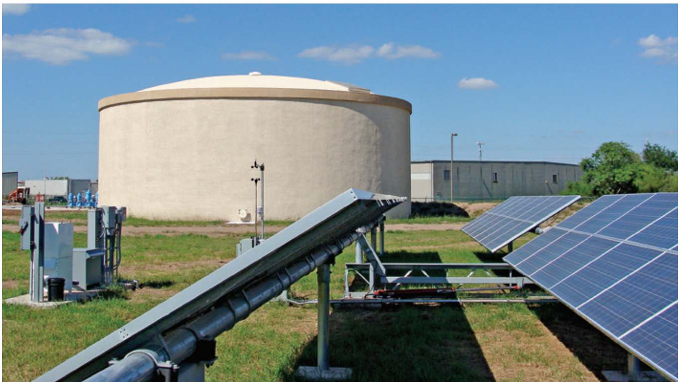
Solar Array at San Benito Water Treatment Plant
