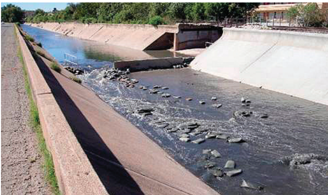
Raw sewage mixed with stormwater and treated with chlorine tablets flows past sandbags in the Nogales Wash used as a bypass for the dilapidated International Outfall Interceptor (IOI). The bypass of sewage into the Nogales Wash in Arizona was undertaken to facilitate repairs of the IOI at the border with Mexico. A dam designed to divert flows back into the IOI was breached by stormwater. Wastewater mixed with stormwater and flowed in an unlined channel as far north as the Santa Cruz River in Rio Rico, 8 miles north of this site (October 28, 2010).
