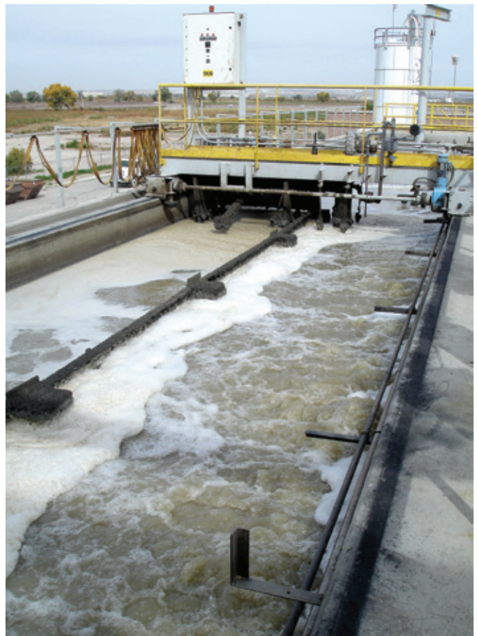
Wastewater Treatment Facility View
