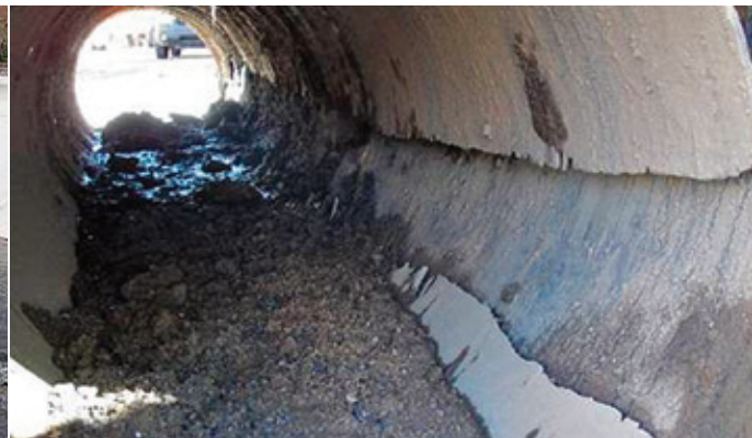
Damaged section of 24" diameter sewer pipe removed at the De Concini Port of Entry. The scour of the wastewater infrastructure in Arizona resulted from the introduction of sediment in Nogales, Sonora. This location is at manhole 1 in Arizona, immediately downstream of the border with Mexico (October 28, 2010).
