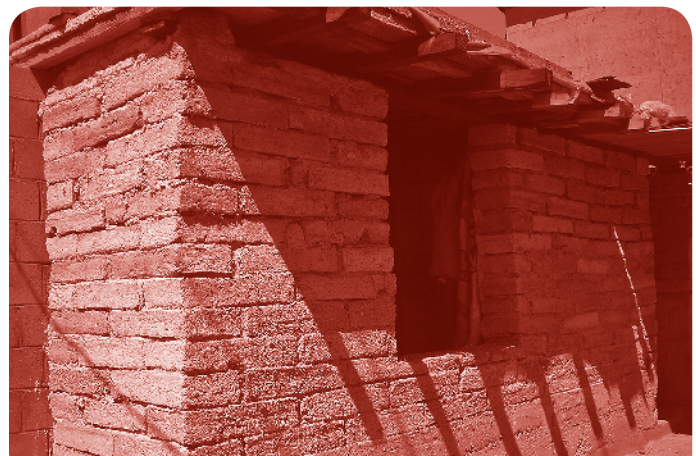
A two room self built fibrous concrete house under construction, Nogales, Sonora.
