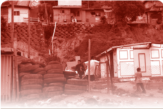
Scrap tires used as foundations for informal housing, Los Laureles Canyon, Tijuana.
