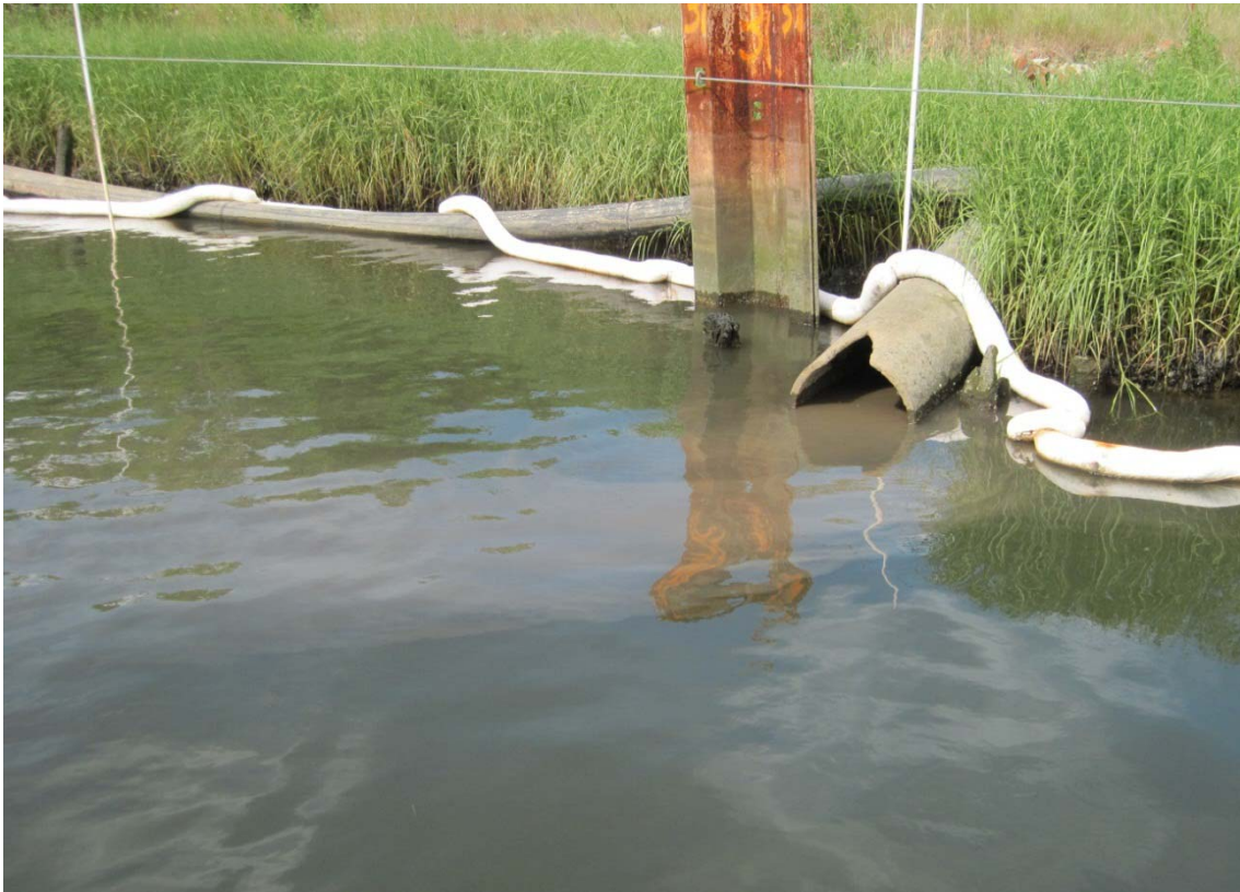
Figure 15. Sediment plume from drainage pipe caused by shore-based construction on 6/27.
