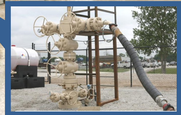
Close-up of Brentwood SWD well in East Fort Worth.
