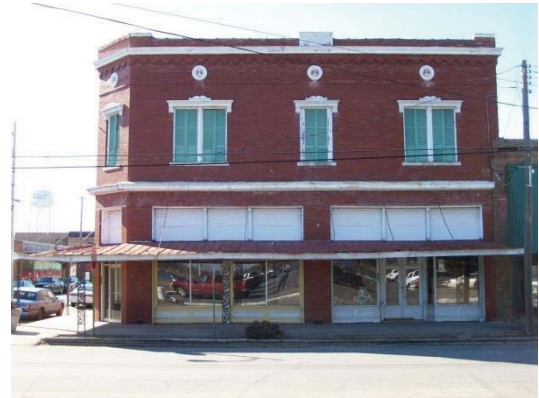
Photos: Historic Lake Villaae. John Tushek Buildina before renovation. Courtesy of Aaron Rubv.
