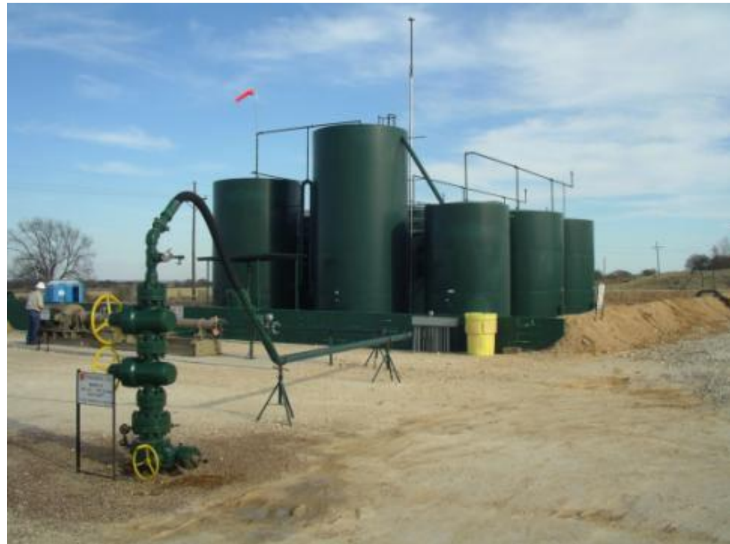
Injection Well and Tank Battery at Commercial Disposal Facility in Texas
