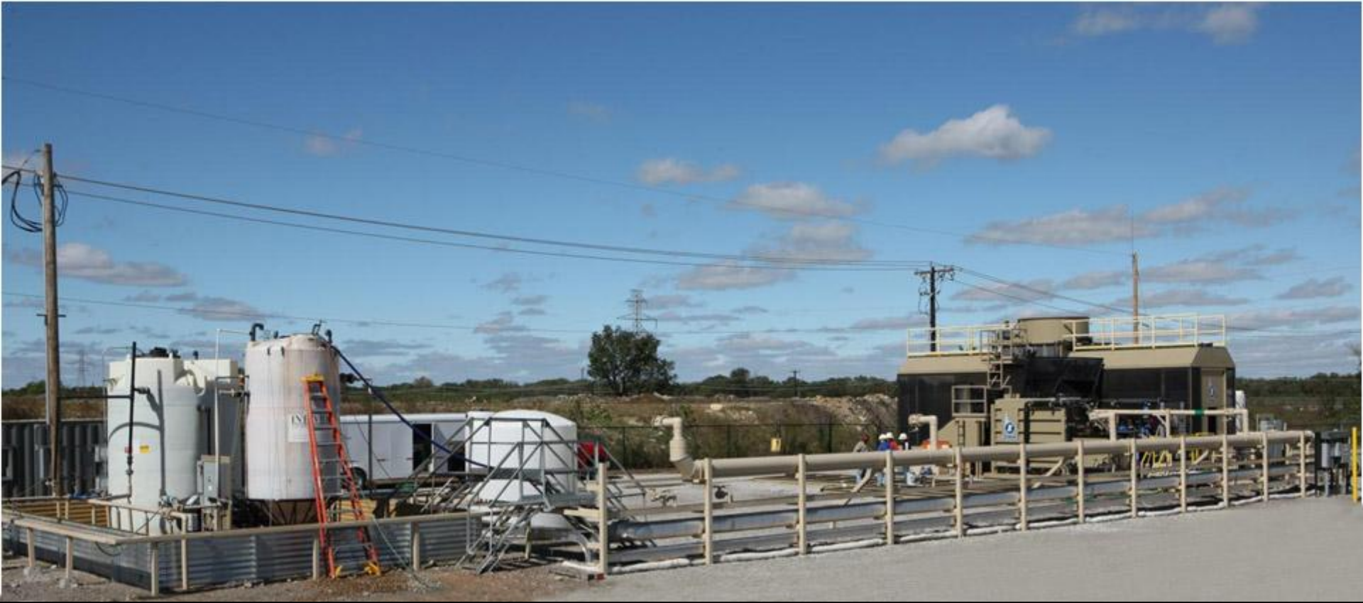
Intevras' EVRAS unit at the Brentwood site in east Fort Worth
