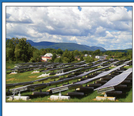
Stafford Hill Solar Farm.
