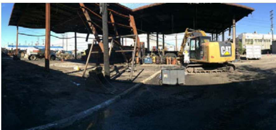
Views from south-center of site before removal on (11/7/2016) and as of today (11/30/2016)
