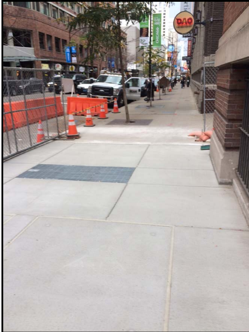
3) Photograph of completed sidewalk taken on 11/28/16 as barricades and fencing were being removed to reopen the sidewalk to pedestrian traffic.
