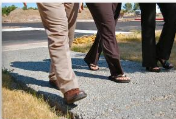
Pervious pavement sidewalk Sioux City, SD
