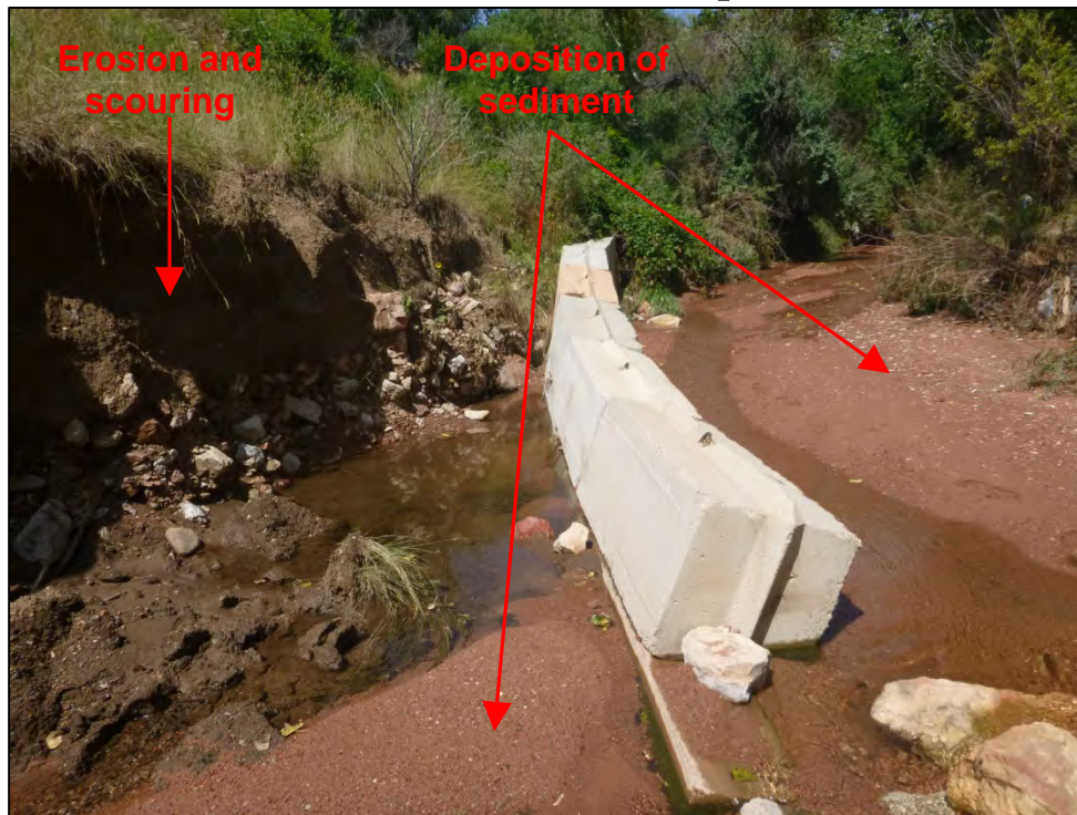
Photograph 23. View, facing upstream, of an unmaintained and deteriorated in-stream concrete bank stabilization measure. Note the deposition of sediment and erosion and scouring of the Douglas Creek channel.
