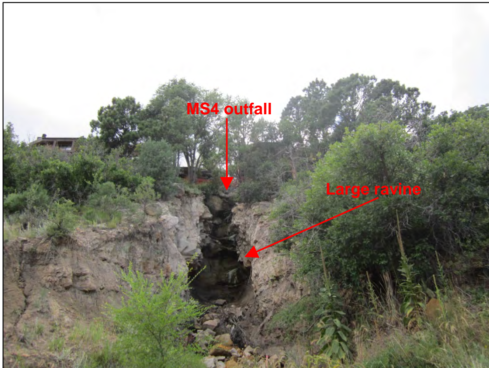
Photograph 58. View of CS – 022 significant erosion and scouring downgradient of the City's MS4 outfall from the Pebblewood at Pinecliff subdivision, including the formation of a large ravine and numerous erosion gullies.
