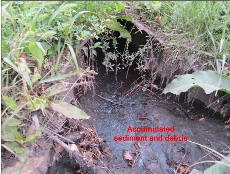
Photograph 83. Close-up view of accumulated sediment and debris at MS4 culvert pipe inlet, shown in Photograph 82.
