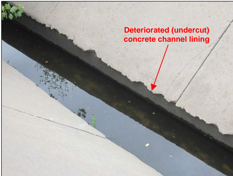
Photograph 74. Close-up view of deteriorated (undercut) concrete channel lining, shown in Photograph 73.
