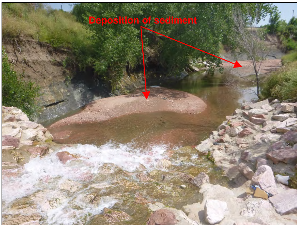
Photograph 42. View of deposition of sediment in N. Douglas Creek located just below the Norfolk Southern railroad bridge. It should be noted that it appeared the railroad may have completed the grouted rip-rap boulder channel stabilization measures in the vicinity of the railroad bridge.
