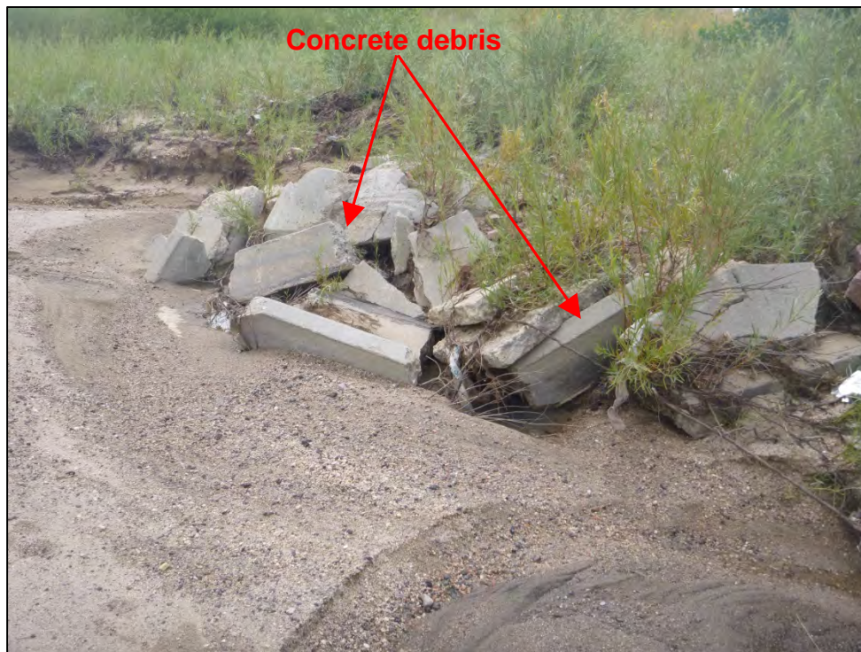
Photograph 120. Close-up view of the concrete debris in the channel, shown in Photograph 119.
