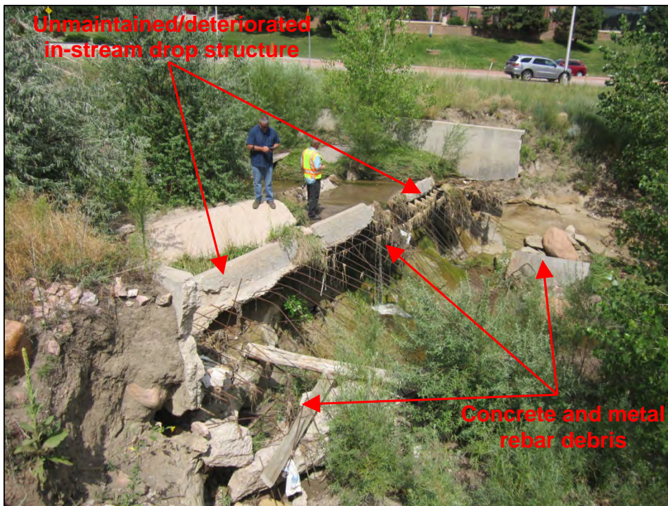
Photograph 46. View of CS – 222 Rockrimmon Channel unmaintained and deteriorated concrete drop structure. Note the significant long-term deterioration including concrete debris and metal rebar scattered about the channel.
