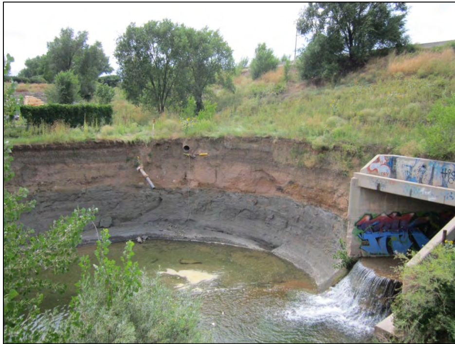
View of significant erosion and scouring of N. Douglas Creek downstream of I-25 box culvert outlet. The vertical dirt embankment was estimated to be approximately a 40 feet high. Portions of the concrete box culvert were present in N. Douglas Creek below the area of this photograph. Also, note that the Creek bed would have been approximately even with the base of the culvert at the time the culvert was constructed and at the time of the 2015 Inspection it appears to be almost 6 feet lower. In addition there is significant undercutting beneath the base of the culvert.
