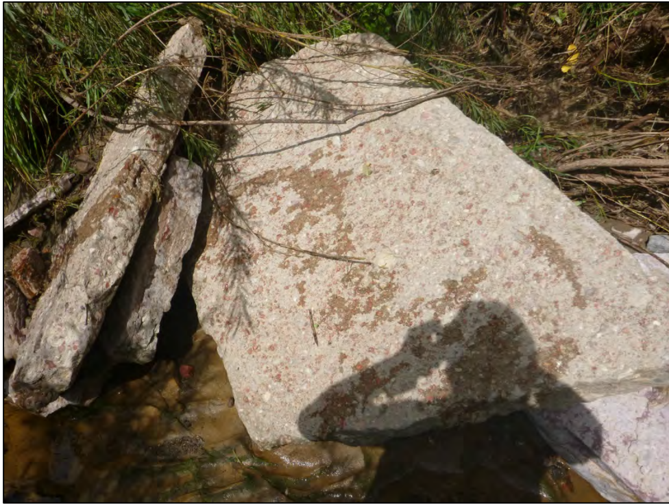
Photograph 51. Close-up view of the concrete debris within the Rockrimmon Channel, shown in Photograph 50.
