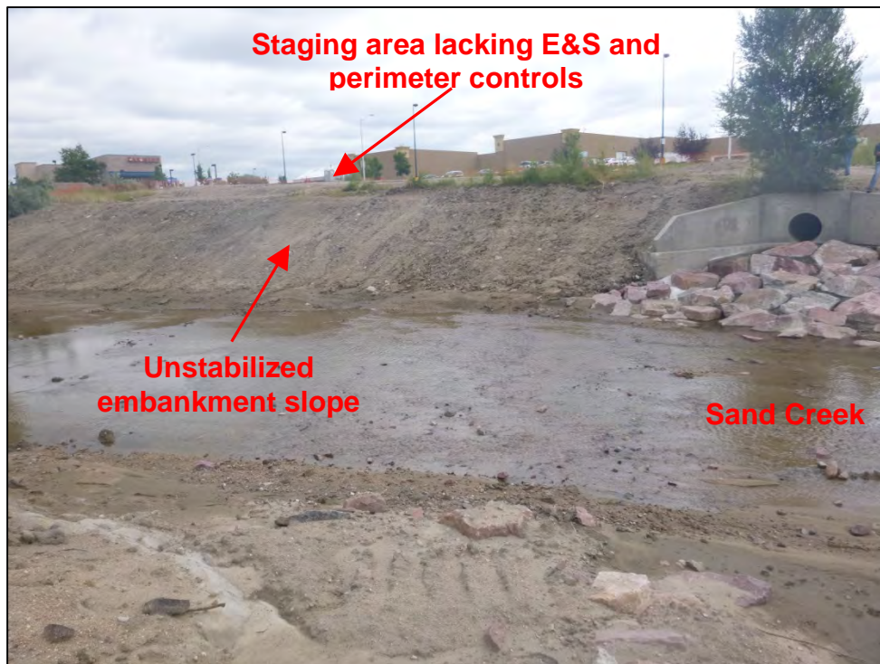
Photograph 98. View of the unstabilized Sand Creek embankment slope located downgradient of the City contractor's staging area for the project. Note that stormwater runoff from this staging area may have been accentuating erosion of this Sand Creek embankment slope.
