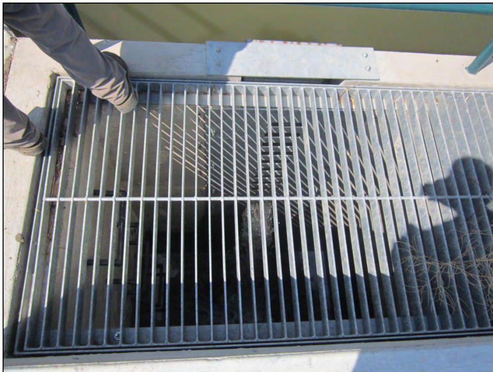
Photograph 142. Close-up view in main detention basin outlet structure. Note that flow was observed flowing through the structure at the time of the inspection.
