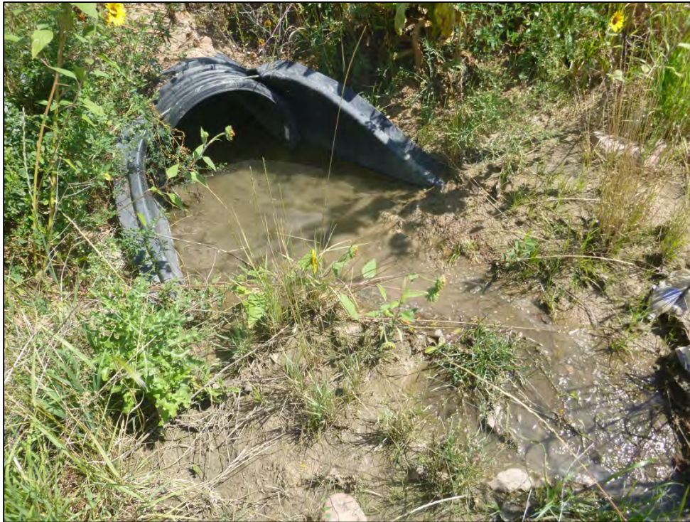
Photograph 12. View of accumulated sediment and vegetative growth at additional inlet pipe to the VA Hospital EDB.
