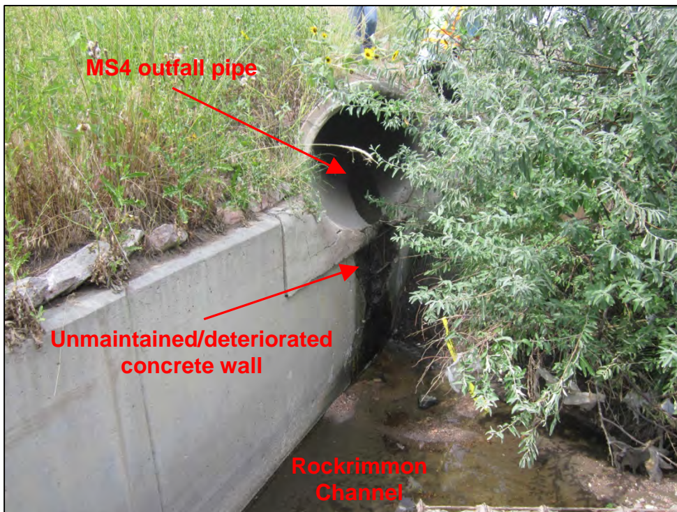
Photograph 54. Additional view of the MS4 outfall pipe, shown in Photograph 53. Note the unmaintained and deteriorated concrete wall below the MS4 outfall pipe and lack of flow dissipation device downgradient of the outfall in Rockrimmon Channel.
