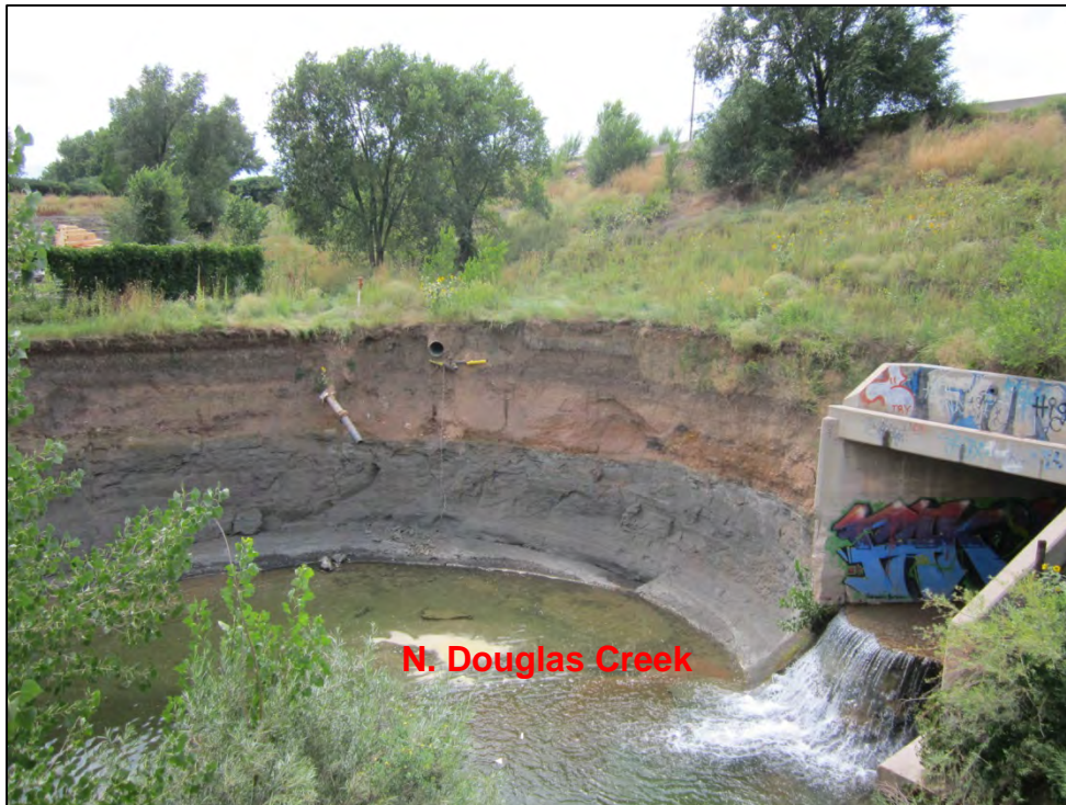
Photograph 35. View of significant erosion and scouring of N. Douglas Creek downstream of I-25 box culvert outlet. The vertical embankment was estimated to be approximately 40 feet high. Portions of the concrete box culvert were present in N. Douglas Creek below the area of this photograph. Also, note that the creek bed would have been approximately even with the base of the culvert at the time the culvert was constructed and at the time of the 2015 Inspection it appears to be almost 6 feet lower. In addition, there was significant undercutting beneath the culvert.
