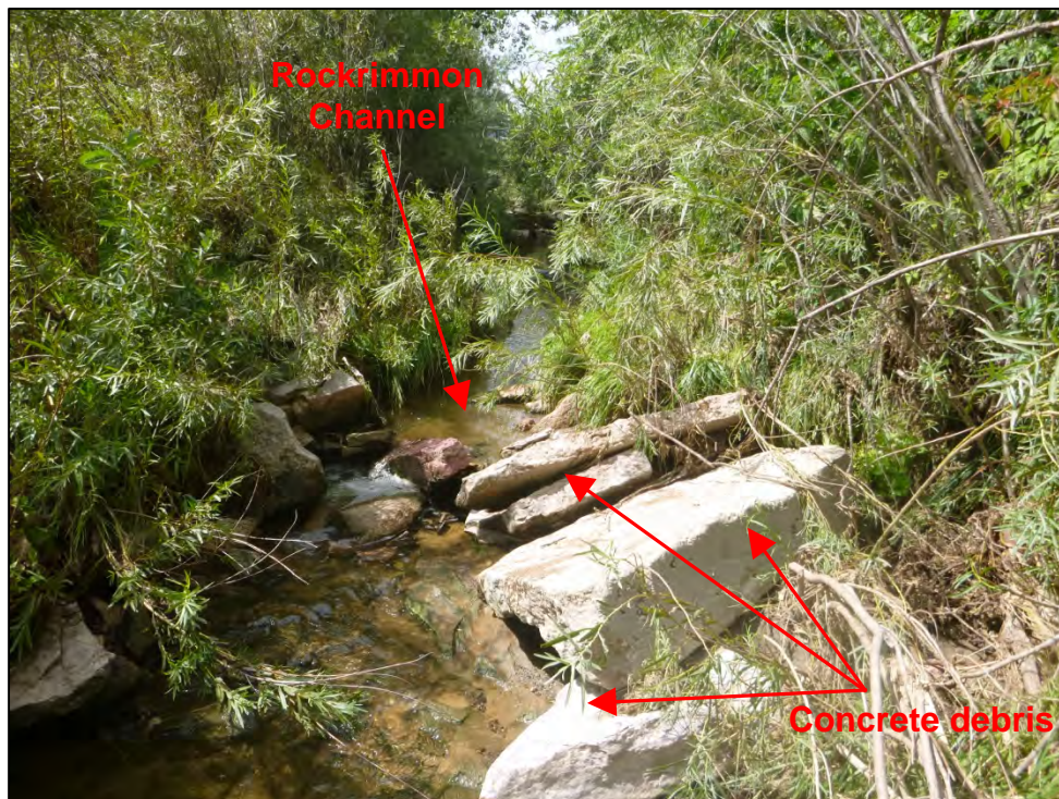
Photograph 50. View of concrete debris scattered about Rockrimmon Channel downstream of the deteriorated concrete drop structure.
