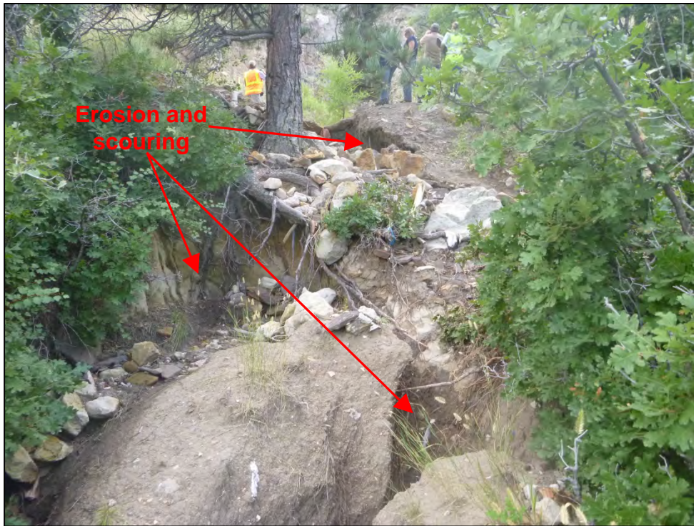
Photograph 61. View of erosion (e.g., gully formation) and scouring on private property located downgradient of MS4 outfall pipe, shown in Photograph 58.
