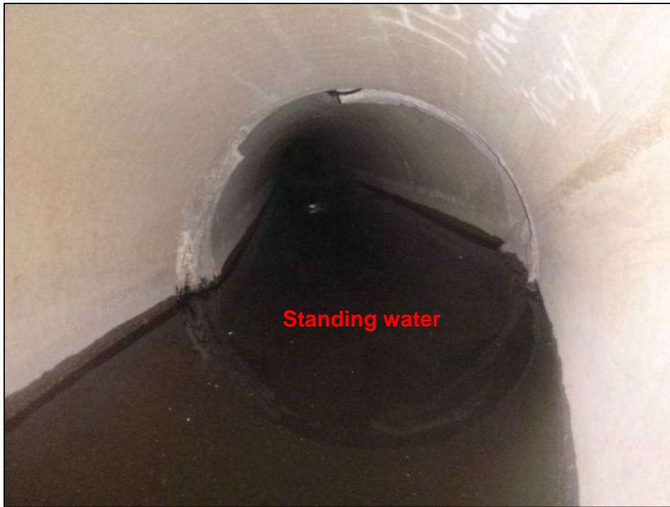
Photograph 65. Close-up view of standing water within the culvert pipe, shown in Photograph 64. Note that this culvert pipe did not appear to have been properly constructed to convey stormwater flow downgradient.
