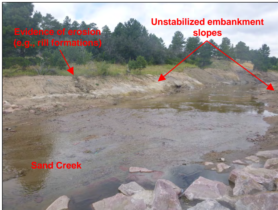
Photograph 94. View of unstabilized Sand Creek embankment slopes with evidence of erosion (e.g., rill formations).
