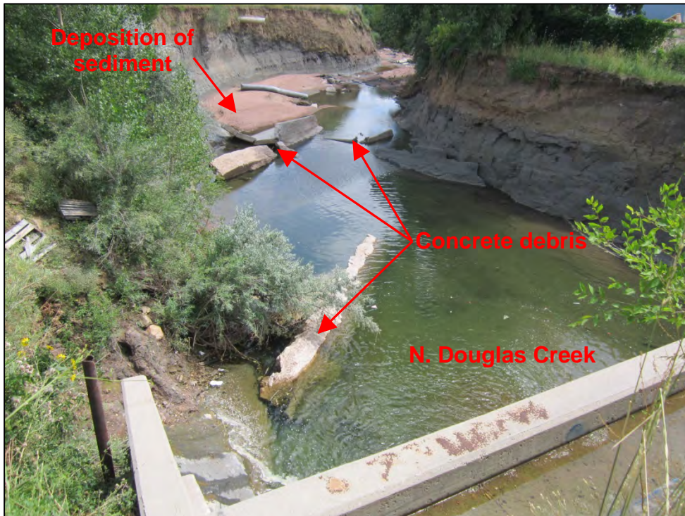
Photograph 36. Additional view of erosion and scouring, concrete debris, and deposition of sediment in the N. Douglas Creek channel downstream of the I-25 box culvert outlet.
