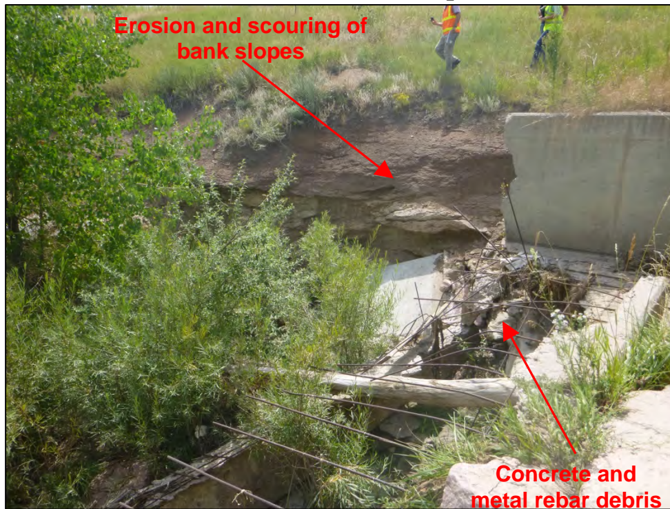
Photograph 49. View of unmaintained and deteriorated in-stream concrete drop structure. Note the concrete and metal rebar debris and erosion and scouring of the Rockrimmon Channel bank slopes.
