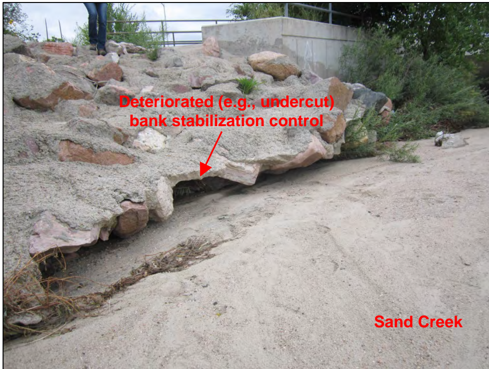
Photograph 81. Close-up view of a deteriorated (e.g., undercut) Sand Creek bank stabilization control. Also note the deposition of sediment in Sand Creek.
