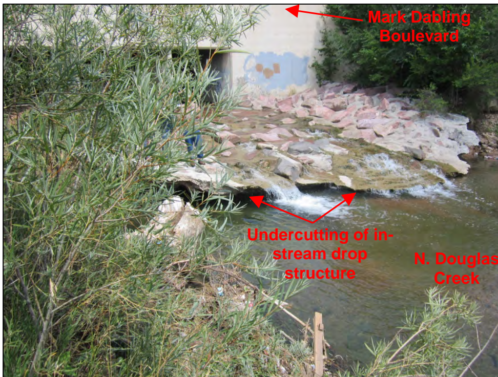
Photograph 32. View of unmaintained in-stream drop structure in N. Douglas Creek downstream of Mark Dabling Boulevard.
