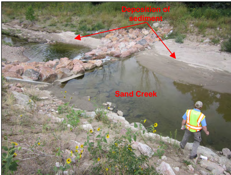
Photograph 103. View of an in-stream engineered drop structure. Note the deposition of sediment upstream and downstream of the structure.
