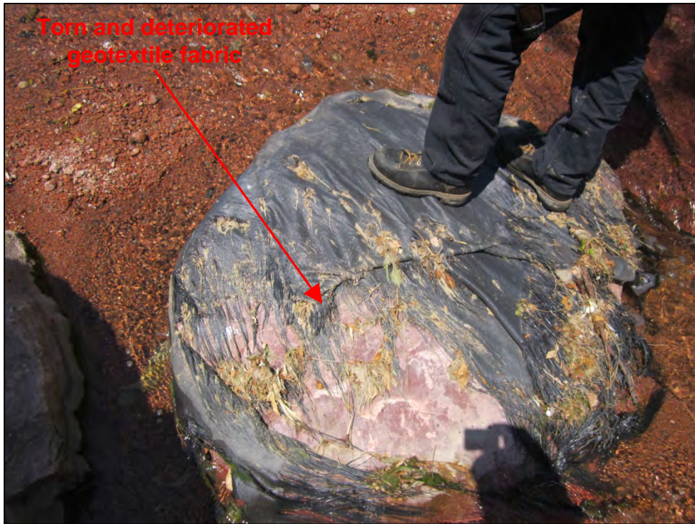
Photograph 27. Close-up view of torn and deteriorated geotextile fabric on in-stream rip-rap. Note that the geotextile appeared to be placed in Douglas Creek along with the rip-rap as part of the recent channel/grade control project.
