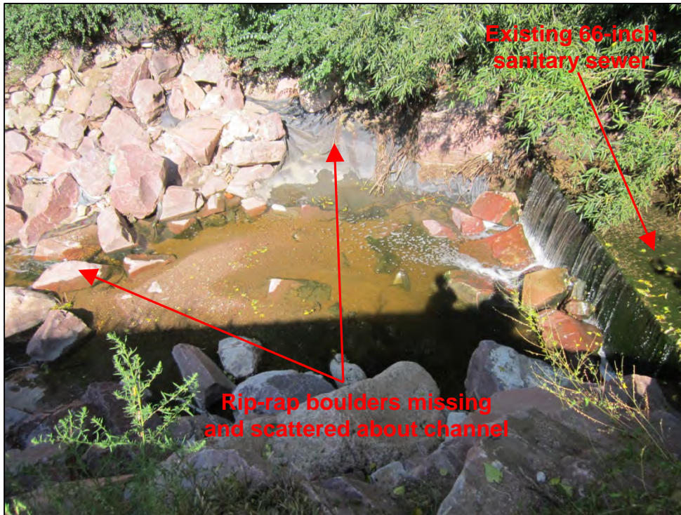
Photograph 1. View of unmaintained rip-rap boulders and channel lining on Shooks Run near the confluence with Fountain Creek.
