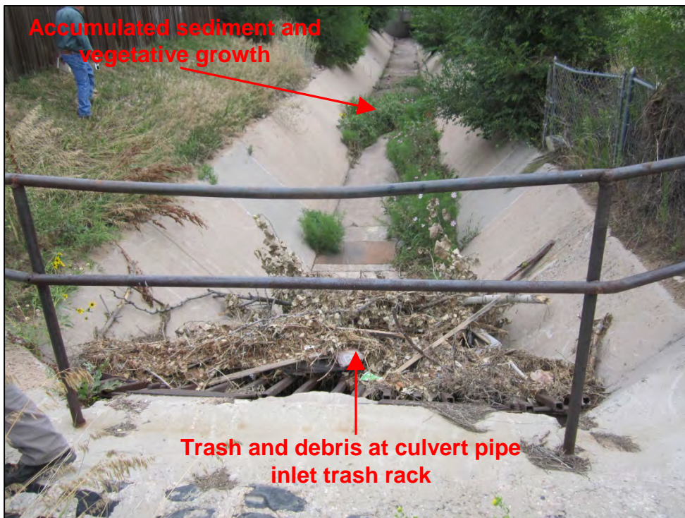
Photograph 66. View, facing upstream, in channel of trash, debris, accumulated sediment and vegetative growth at the culvert pipe inlet trash rack and within the concrete lined channel itself.
