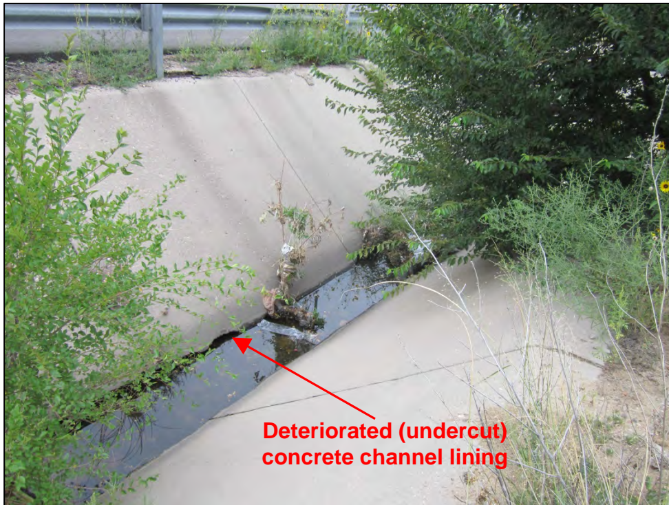
Photograph 73. View of unmaintained/deteriorated (undercut) concrete channel lining.
