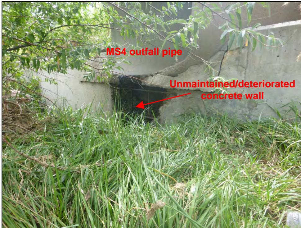
Photograph 55. Close-up view of the unmaintained and deteriorated concrete wall below the MS4 outfall pipe, shown in Photograph 54.
