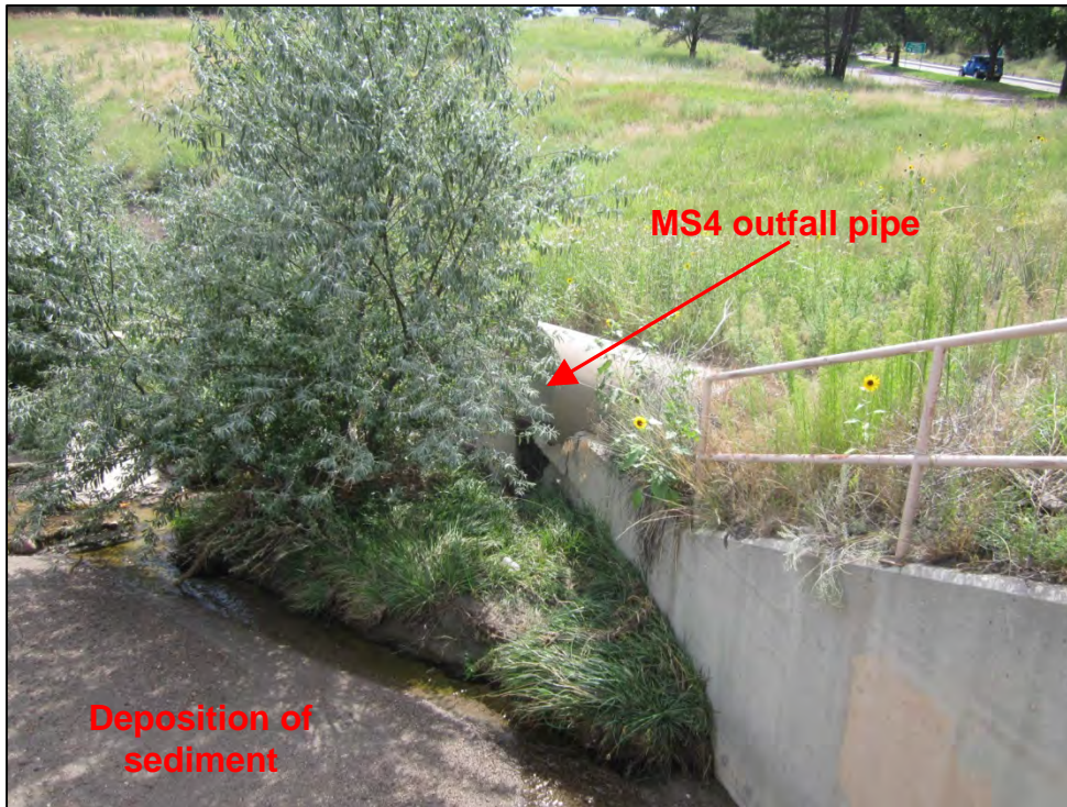
Photograph 53. View of the MS4 outfall pipe to Rockrimmon Channel near the intersection of Rockrimmon Boulevard and Pro Rodeo Drive. Note the deposition of sediment.
