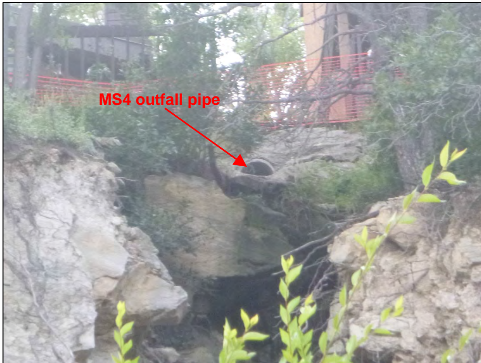
Photograph 60. Additional close-up view of the MS4 outfall pipe and ravine/cliff area adjacent to the outfall.
