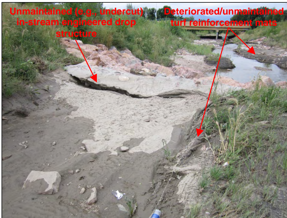
Photograph 106. View of deteriorated and unmaintained turf reinforcement mat BMPs implemented in Sand Creek. Also note the unmaintained (e.g., undercut) grouted rip-rap boulder in-stream engineered drop structure.
