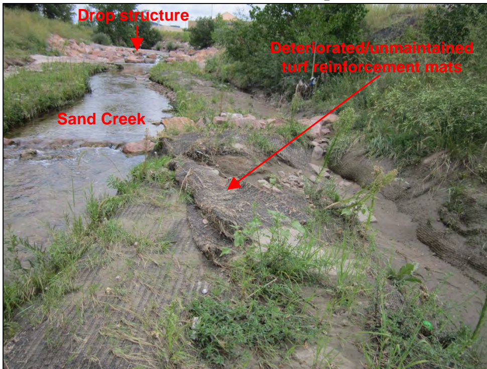
Photograph 105. Additional view of deteriorated and unmaintained turf reinforcement mat BMPs implemented in Sand Creek downstream of an engineered in-stream drop structure, shown in Photograph 103.
