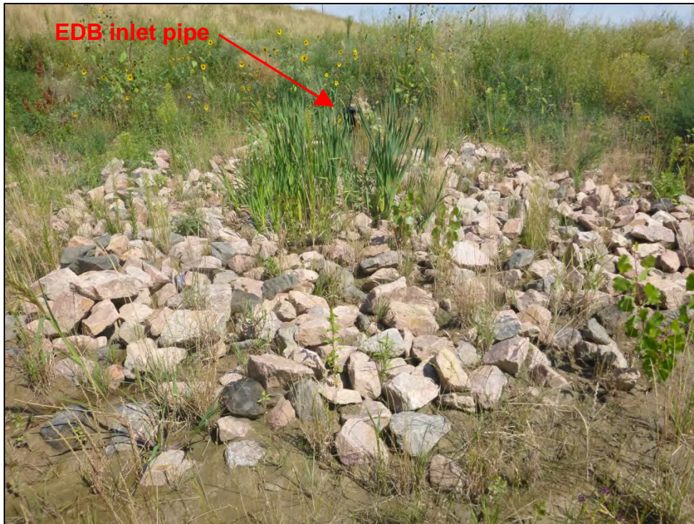
Photograph 13. View of vegetative growth in flow dissipation (rip-rap) device downgradient of the inlet pipe, shown in Photograph 12.
