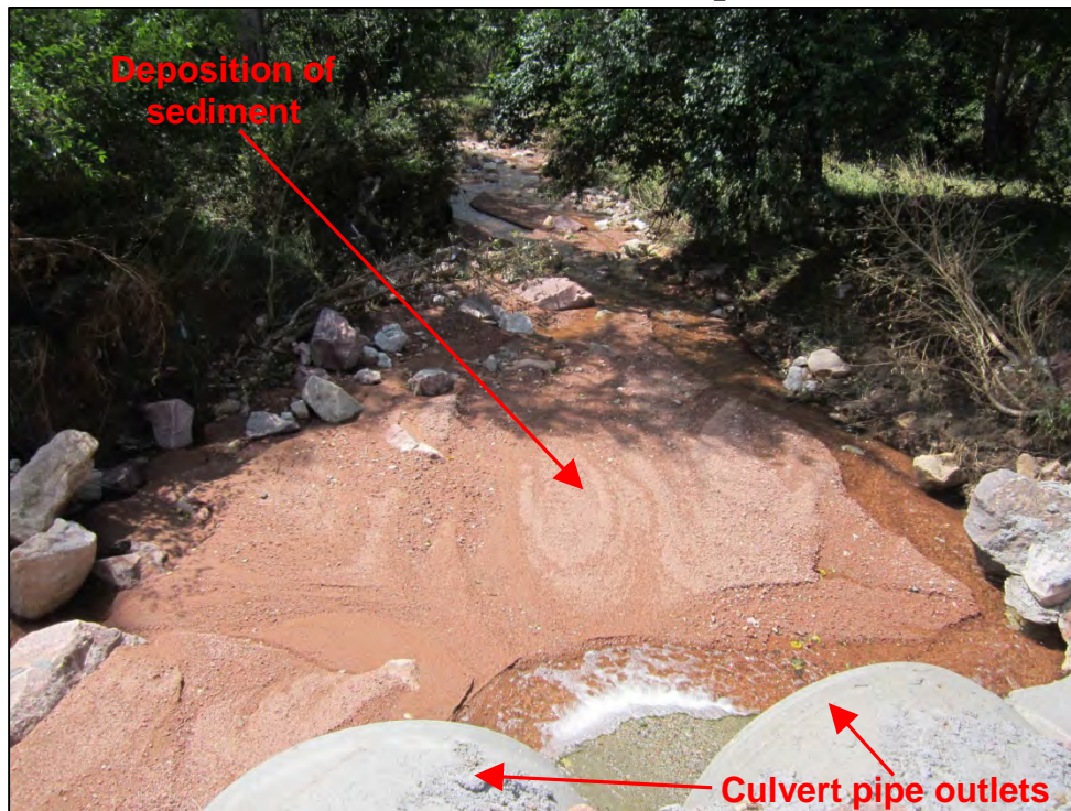
Photograph 21. View facing downstream of Douglas Creek low water crossing. Note the deposition of sediment within the Douglas Creek channel downstream of the low water crossing culvert pipe outlets.
