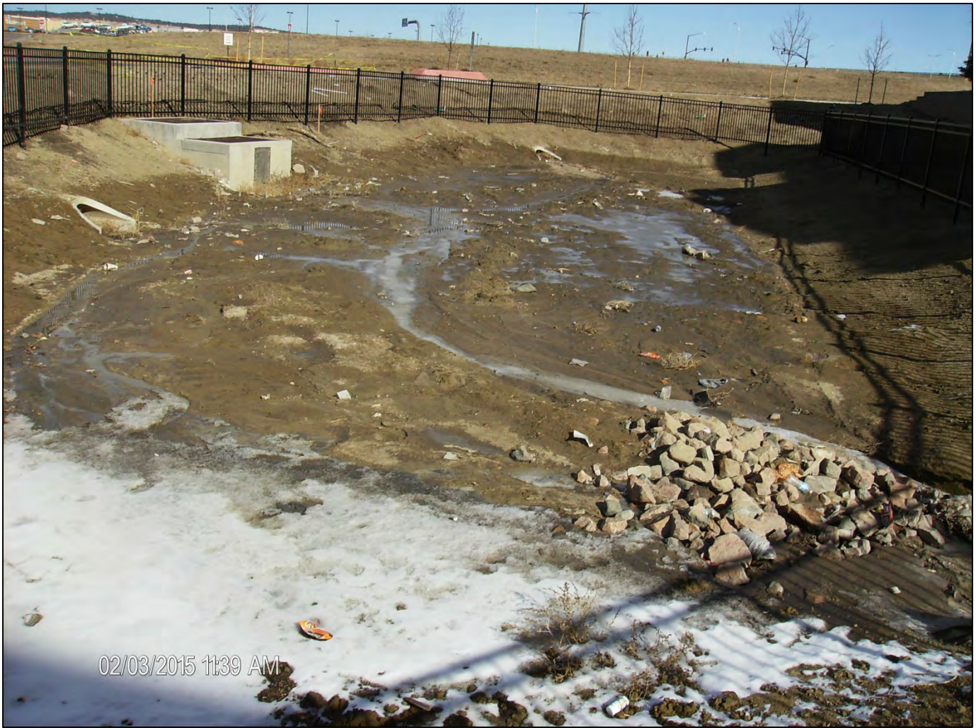
Exhibit 19. City provided photograph of ID – 070 Woodmen Ridge Apartments EDB, dated February 3, 2105. Note that the EDB was unstabilized and contained accumulated sediment and debris.
