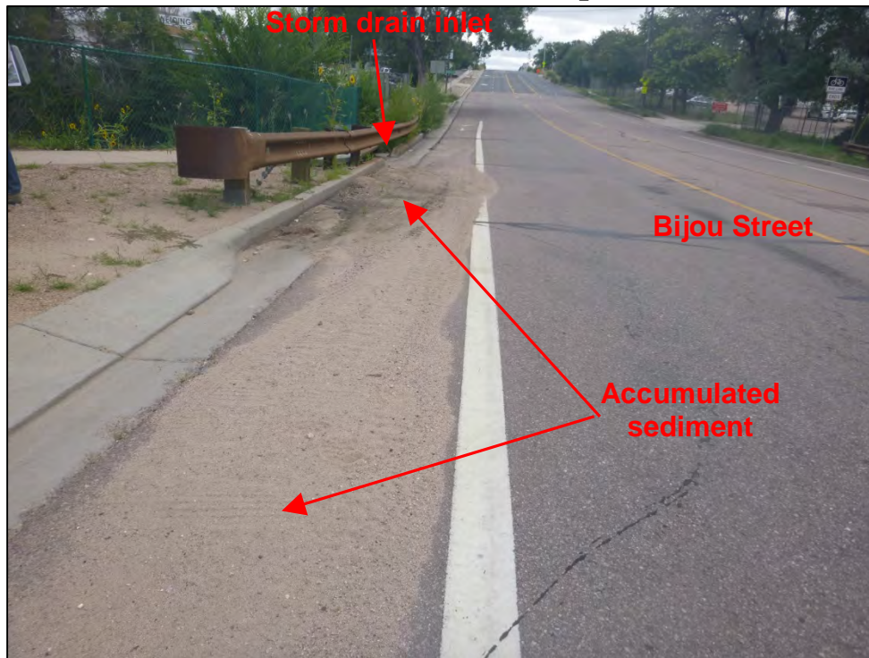
Photograph 89. View of accumulated sediment on roadway adjacent to a storm drain inlet that drains directly to Spring Creek.
