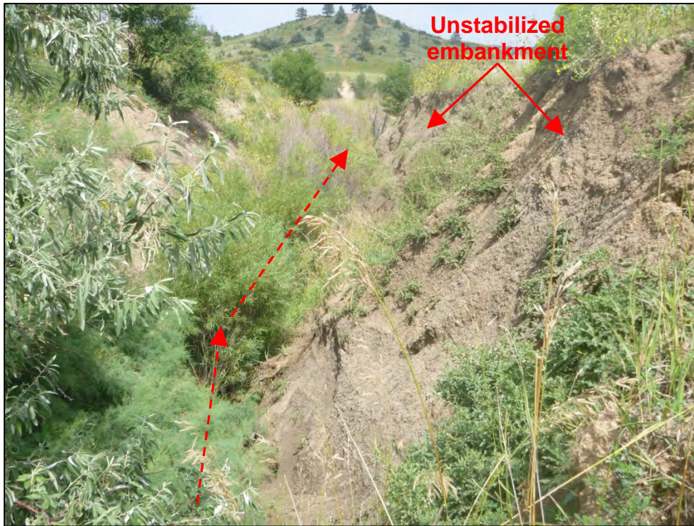
Photograph 45. Close-up view of the drainage channel and unstabilized embankment downgradient of the storm drain outlet for the storm drain shown in Photograph 43.
