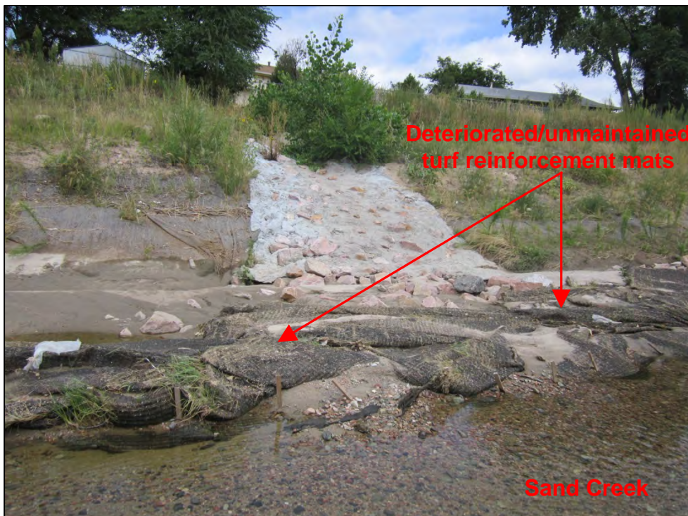
Photograph 108. View of deteriorated and unmaintained turf reinforcement mat BMPs implemented in Sand Creek. Note the in-stream BMPs had been implemented below a grouted rip-rap stormwater conveyance channel (i.e., potential area of concentrated flow) outfall.
