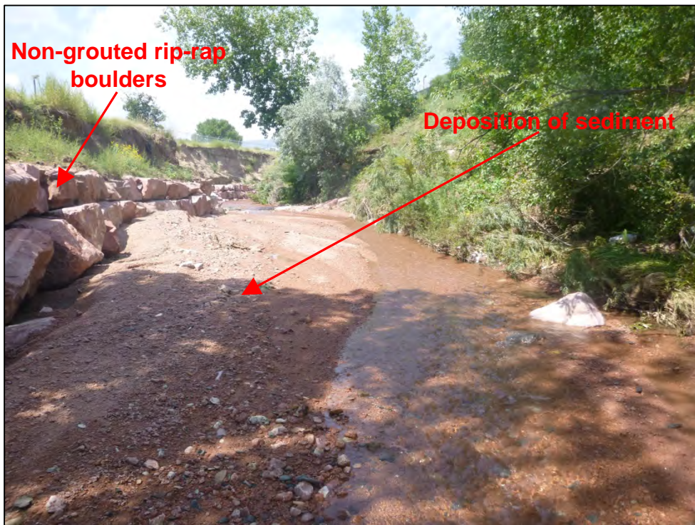
Photograph 28. View, facing upstream, of significant deposition of sediment within Douglas Creek adjacent to the stream bank stabilization project.
