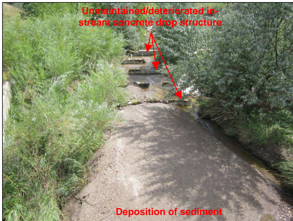
Photograph 48. View of deposition of sediment above the deteriorated in-stream drop structure shown in Photograph 47, above.
