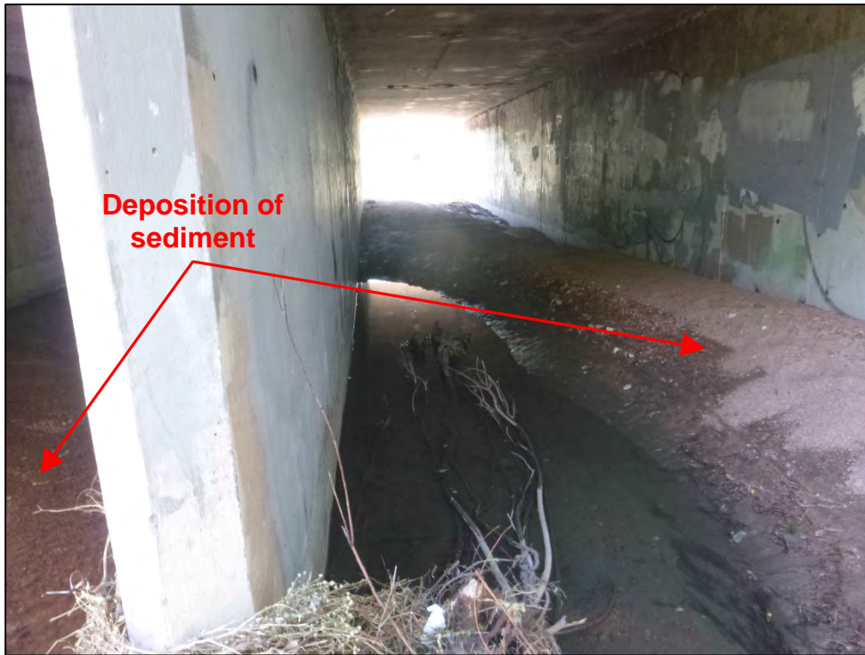
Photograph 31. Close-up view of significant deposition of sediment in the box culvert under Mark Dabling Boulevard on N. Douglas Creek.
