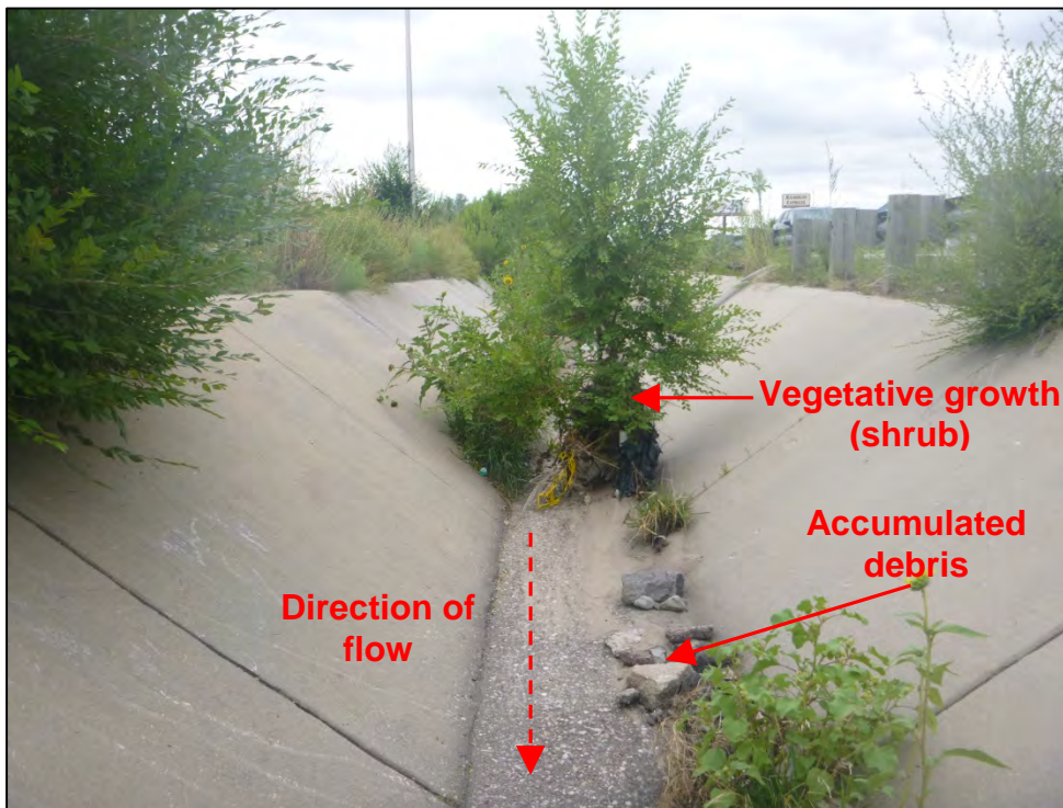
Photograph 78. Close-up view of vegetative growth (e.g., shrubs) and accumulated debris in the channel.
