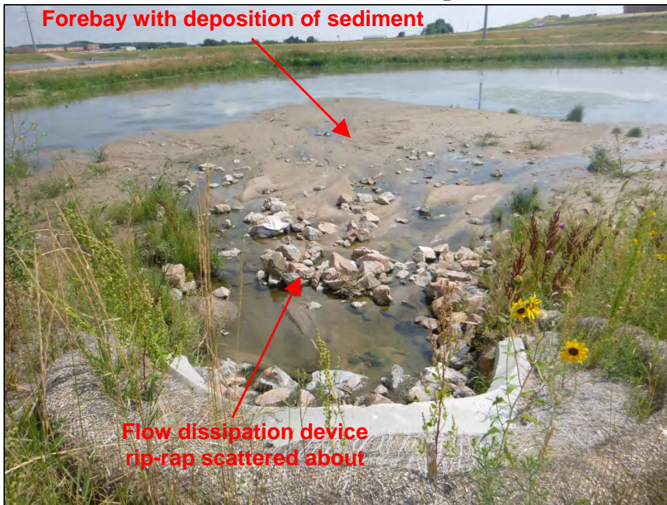
Photograph 135. View of second forebay and inlet with deposition of sediment and unmaintained flow dissipation device (e.g., rip-rap scattered in forebay).
