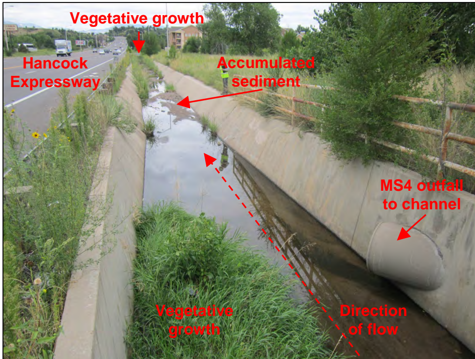
Photograph 76. View, facing downstream, of concrete lined MS4 conveyance channel located along Hancock Expressway near Astrozon Boulevard. Note the vegetative growth and accumulated sediment in the channel.
