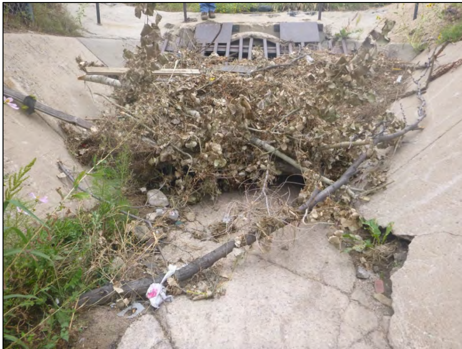
View of CS – 060 Hancock Expressway Drainage channel. View in channel of trash, debris, accumulated sediment, vegetative growth, and deteriorated concrete channel lining at the culvert pipe inlet trash rack and within the concrete lined channel itself.
