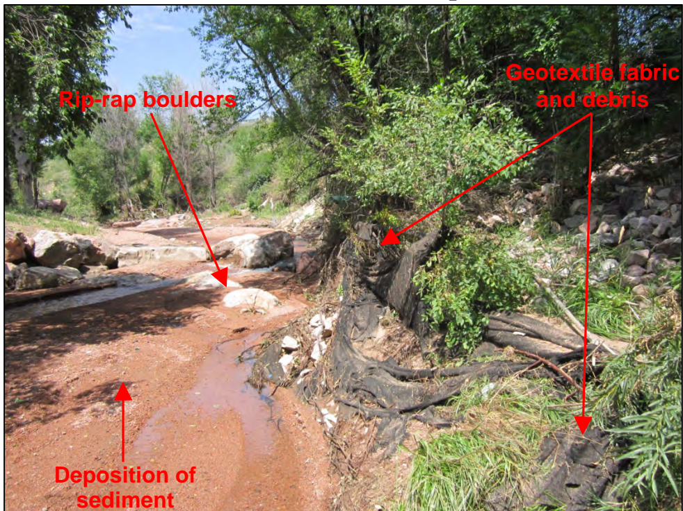
Photograph 29. View, facing upstream, of Douglas Creek. Note the geotextile fabric, debris, and rip-rap boulders scattered about the channel. Also note the deposition of sediment in the channel.
