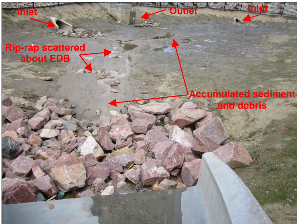
Photograph 129. View of accumulated sediment and debris at additional inlet and forebay. Also note the rip-rap scattered about the EDB.
