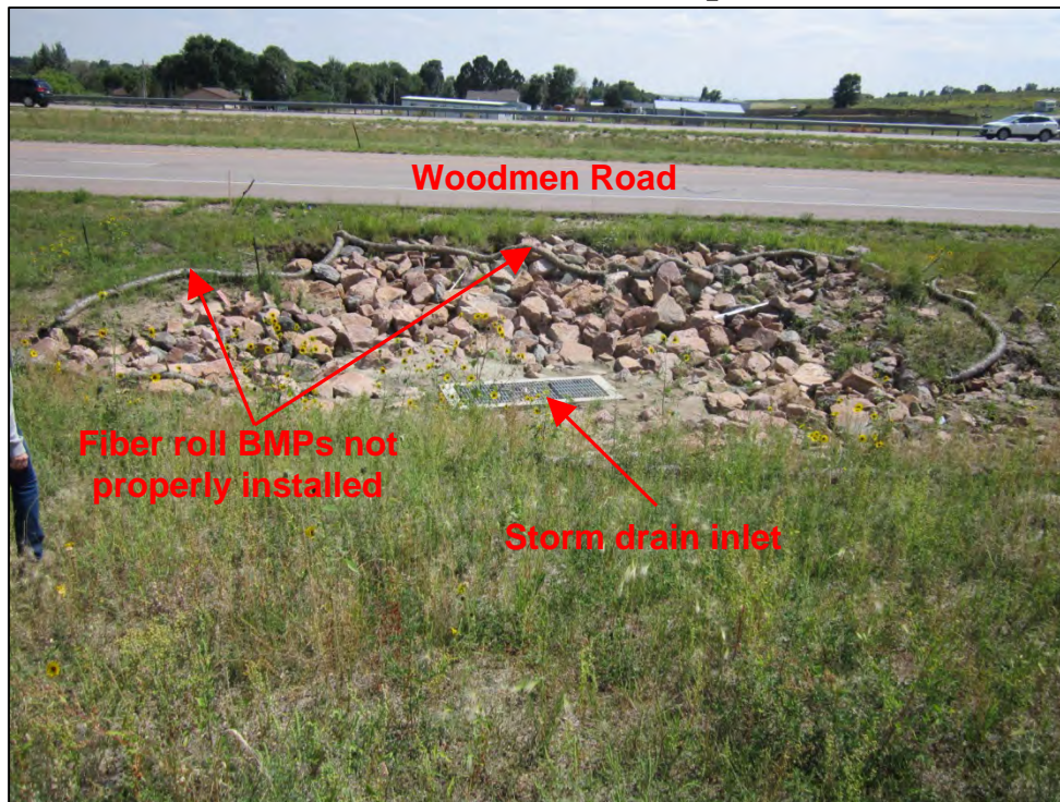
Photograph 143. View of storm drain inlet with fiber roll BMPs not properly installed (e.g., not staked or entrenched, placed on rip-rap) located adjacent to Woodmen Road. It should be noted that this storm drain inlet is inline with the main detention basin outlet structure conveyance pipe.
