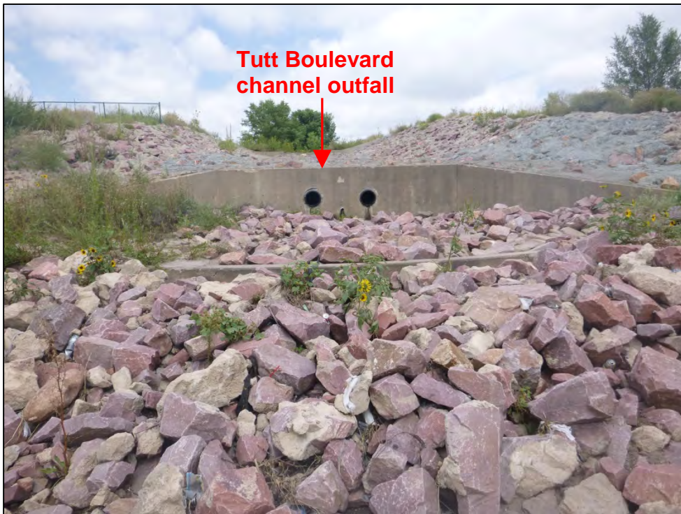
Photograph 116. View, facing upstream, of Tutt Boulevard channel outfall to the Sand Creek Detention Basin No. 1, shown in Photograph 111.
