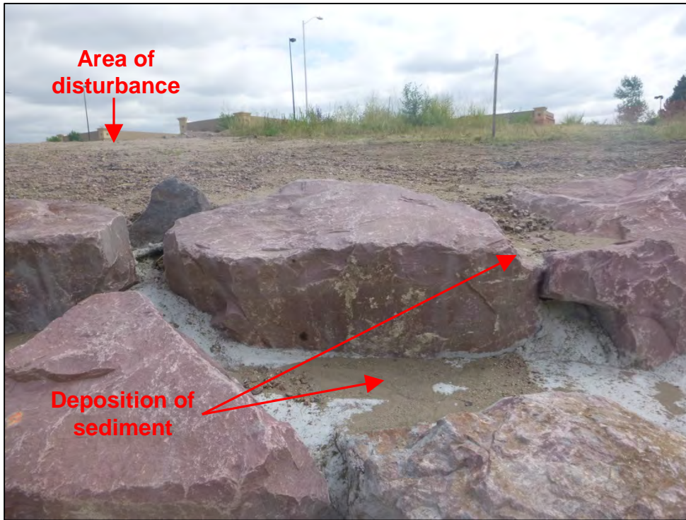
Photograph 101. View, facing upgradient, toward the unstabilized area of disturbance (i.e., staging area) and close-up of the evidence of the previous release and deposition of sediment to the Sand Creek embankment slope.
