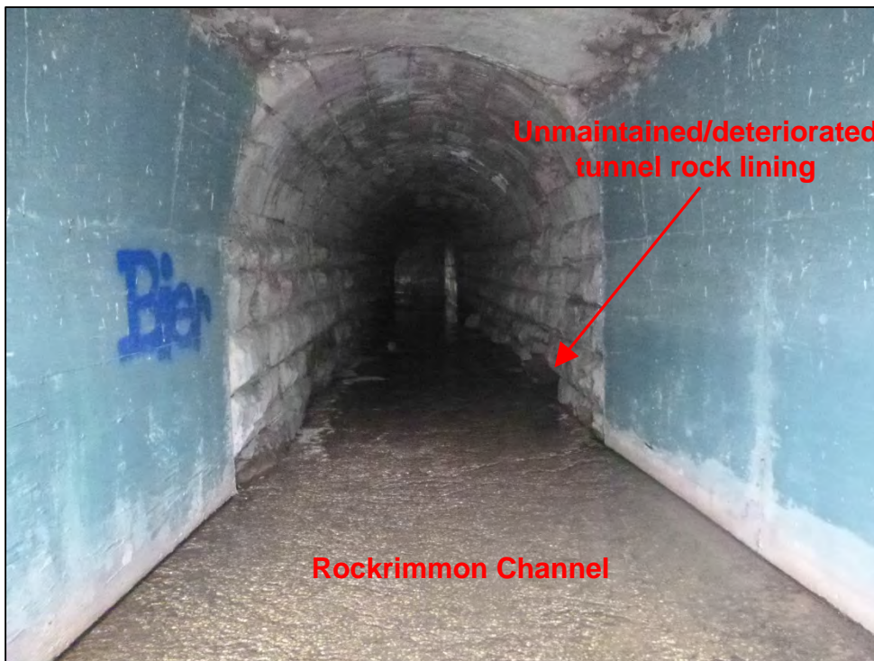
Photograph 56. View of Rockrimmon Channel conveyance tunnel under Norfolk Southern railroad bridge and Mark Dabbling Boulevard. Note the unmaintained and deteriorated tunnel rock lining.
