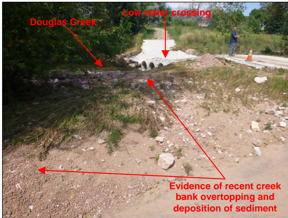
Photograph 19. View of recent evidence of creek bank and culvert pipe overtopping with deposition of sediment.
