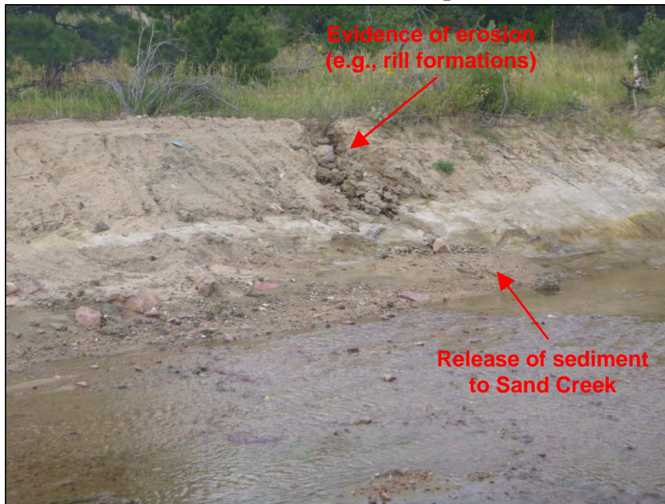
Photograph 95. Close-up view of the unstabilized Sand Creek embankments slopes with evidence of erosion (e.g., rill formations) and a release of sediment to Sand Creek.
