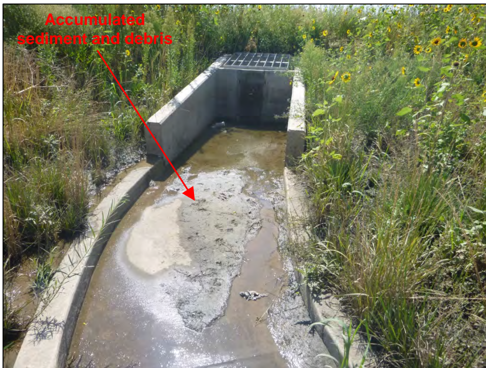
Photograph 14. View of accumulated sediment and debris within the trickle channel and micropool adjacent to the outlet structure. Also note the dense vegetative growth adjacent to the EDB outlet structure.
