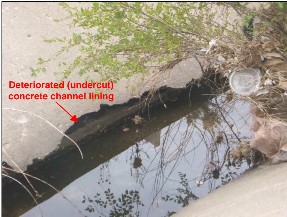
Photograph 75. Additional close-up view of deteriorated (undercut) concrete channel lining.
