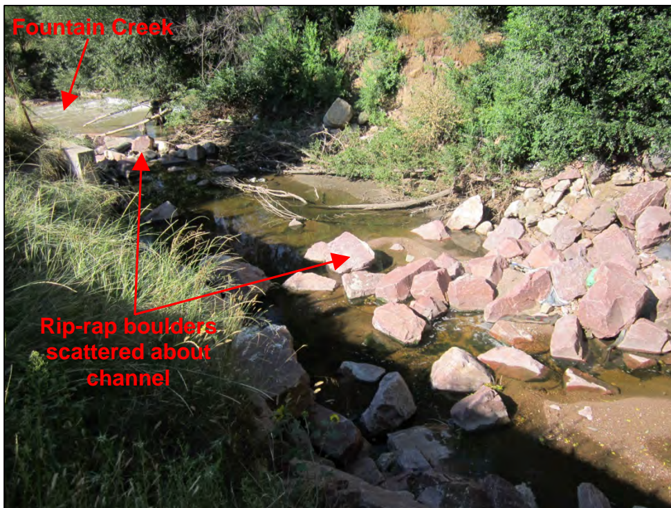
Photograph 2. View of rip-rap boulders and debris scattered throughout the Shooks Run channel near the confluence with Fountain Creek.
