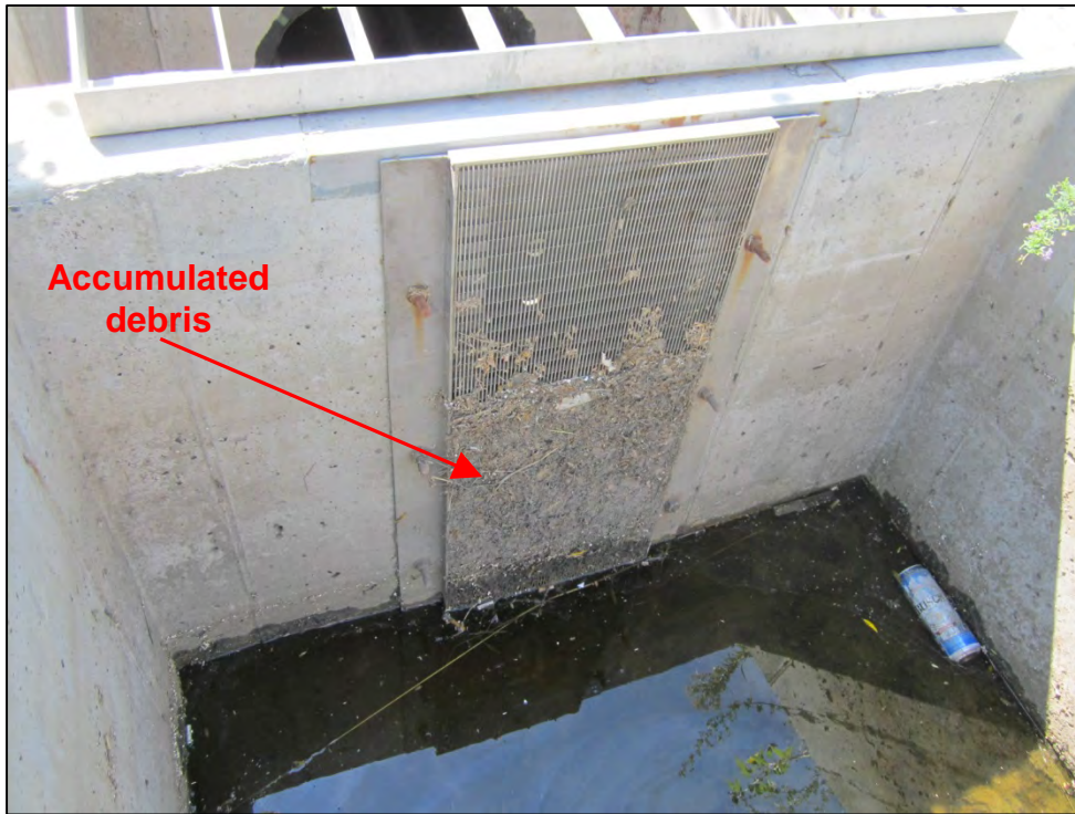
Photograph 15. Close-up view of accumulated debris on the outlet structure screen orifice plate.
