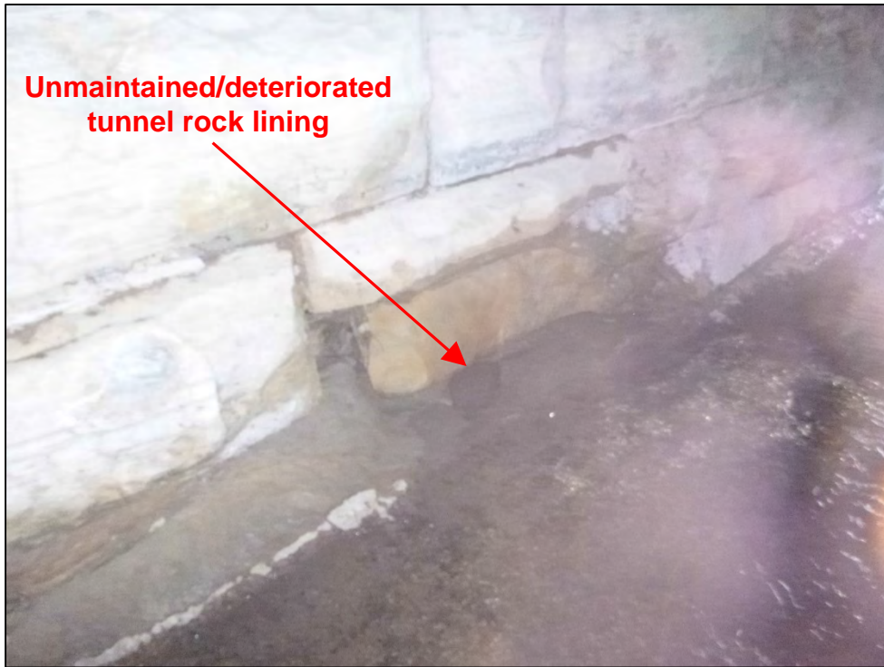
Photograph 57. Close-up view of the unmaintained and deteriorated tunnel rock lining.
