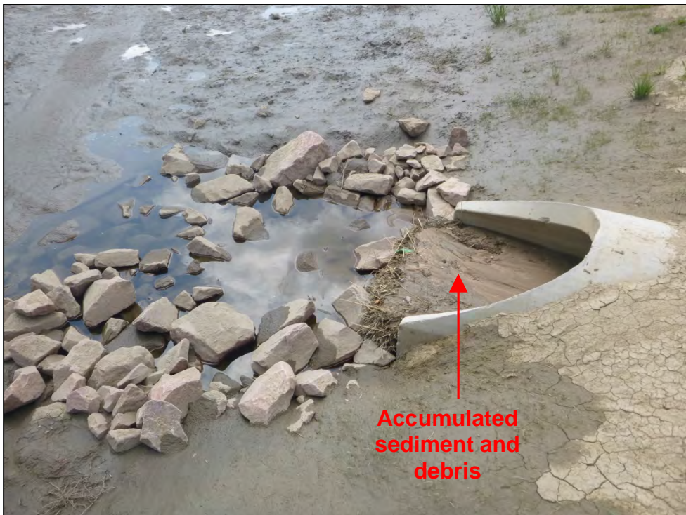
Photograph 128. View of accumulated sediment and debris at an additional inlet and associated forebay.
