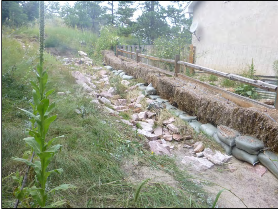
View of evidence of previous stormwater runoff and erosion adjacent to the Chiramonte private property. The City had installed straw bales and sandbag BMPs along the property boundary.
