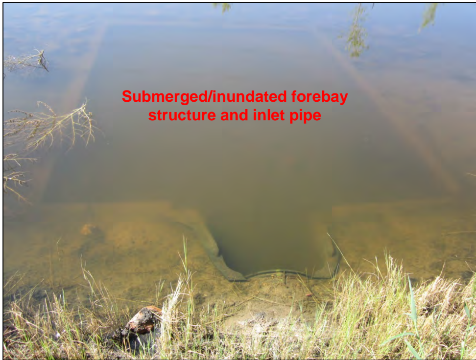
Photograph 7. Close-up view of the EDB submerged/inundated northeast inlet pipe and forebay structure, shown in Photographs 5 and 6. Note that the elevation of this inlet pipe and forebay was approximately one foot lower than the EDB outfall pipe.
