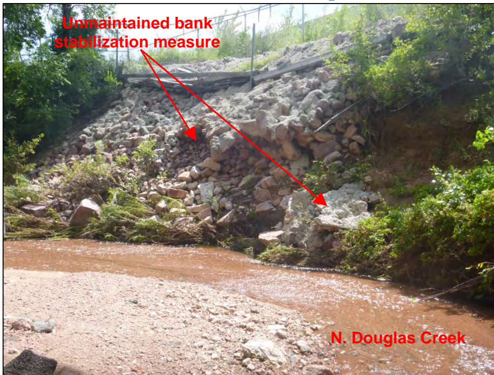
Photograph 41. View of unmaintained bank stabilization measure located just upstream of Norfolk Southern railroad bridge.
