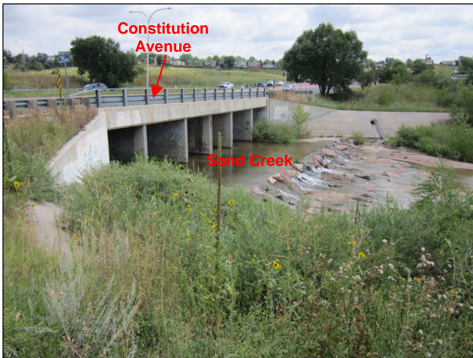
Photograph 124. View of detention basin box culvert outlet to Sand Creek downgradient of the outlet structure at Constitution Avenue.
