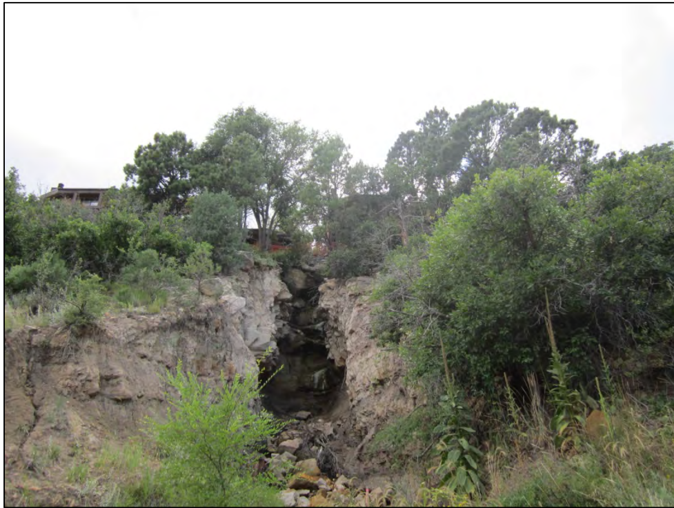
View of CS – 022 significant erosion and scouring downgradient of the City’s MS4 outfall from the Pebblewood at Pinecliff subdivision, including the formation of a large ravine and numerous erosion gullies.
