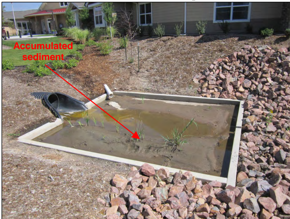
Photograph 9. View of accumulated sediment and debris in the western inlet forebay. Note that this did not appear to have been identified on City inspection reports. Also note that the western inlet forebay had not been adequately maintained.
