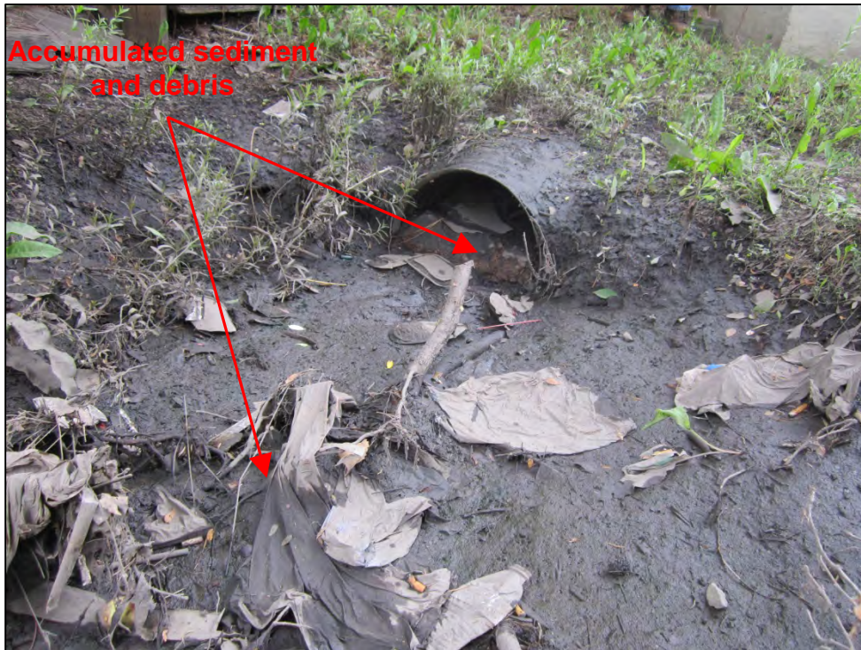
Photograph 85. Close-up view of accumulated sediment and debris at MS4 culvert pipe outlet, shown in Photograph 84. Note the CMP pipe appeared to be at approximately 50 percent capacity due to accumulated sediment and debris within the pipe.
