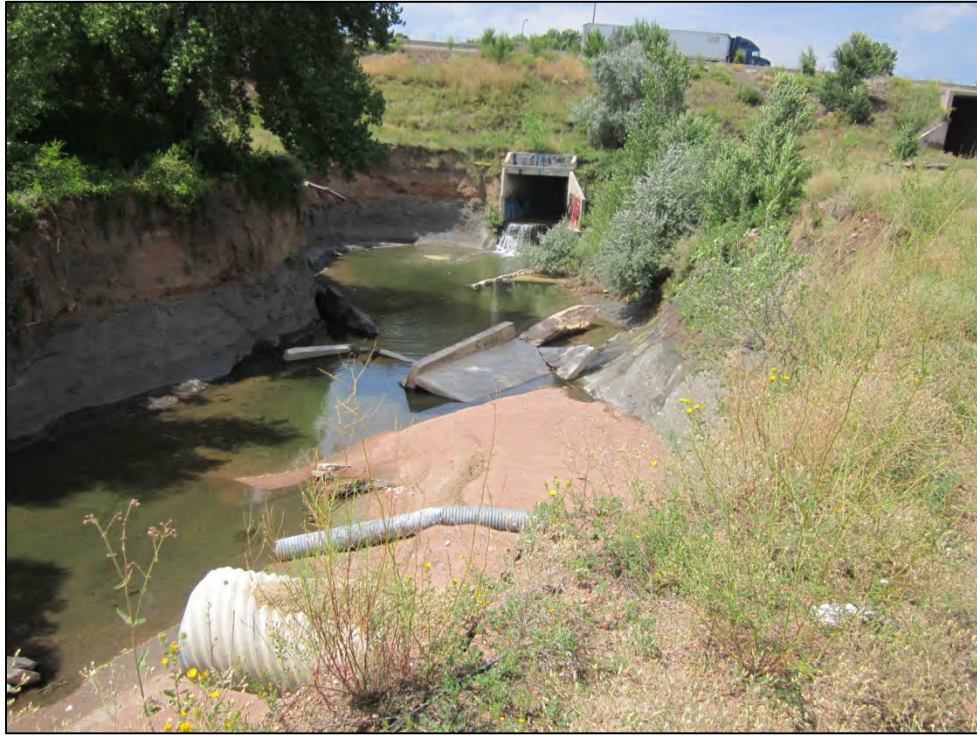
View, facing upstream and toward I-25, of erosion and scouring, concrete debris, old CMP culvert pipe, and sediment deposition in North Douglas Creek.
