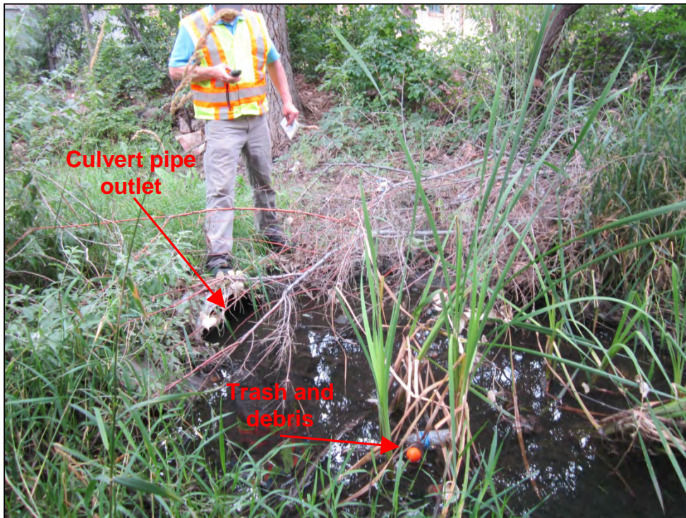
Photograph 86. View of second culvert CMP pipe outlet into what appeared to be a wetland area behind the residences. Note the standing water and trash and debris.
