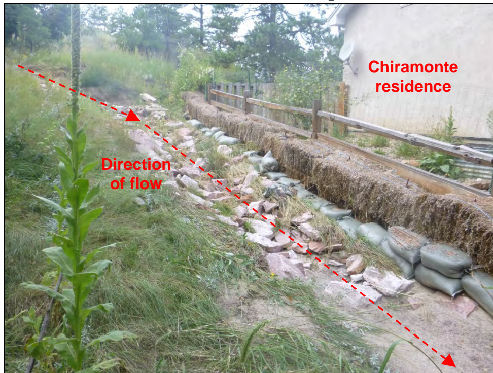
Photograph 63. View of evidence of previous stormwater runoff and erosion adjacent to the Chiramonte private property. Note the City had implemented straw bales and sand bag BMPs along the property boundary.
