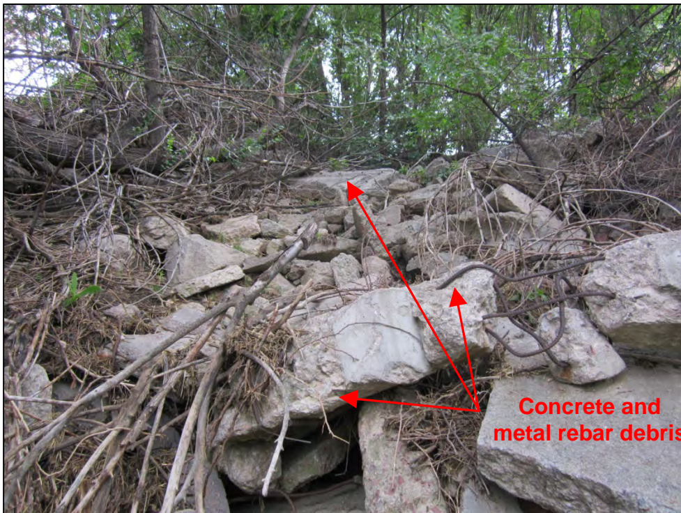
Photograph 52. Additional view of concrete and metal rebar debris in the Rockrimmon Channel located downstream of the unmaintained drop structure.
