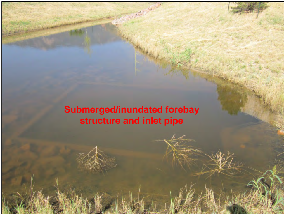
Photograph 8. Additional close-up view of the submerged/inundated northeast inlet pipe and forebay structure, shown in Photograph 7. Note the forebay design (i.e., energy dissipation and sediment removal) was impaired due to the elevations of these structures being approximately one foot lower than the outfall pipe invert.
