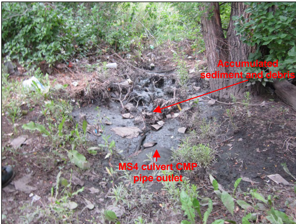
Photograph 84. View of accumulated sediment and debris at the City MS4 culvert pipe outlet.
