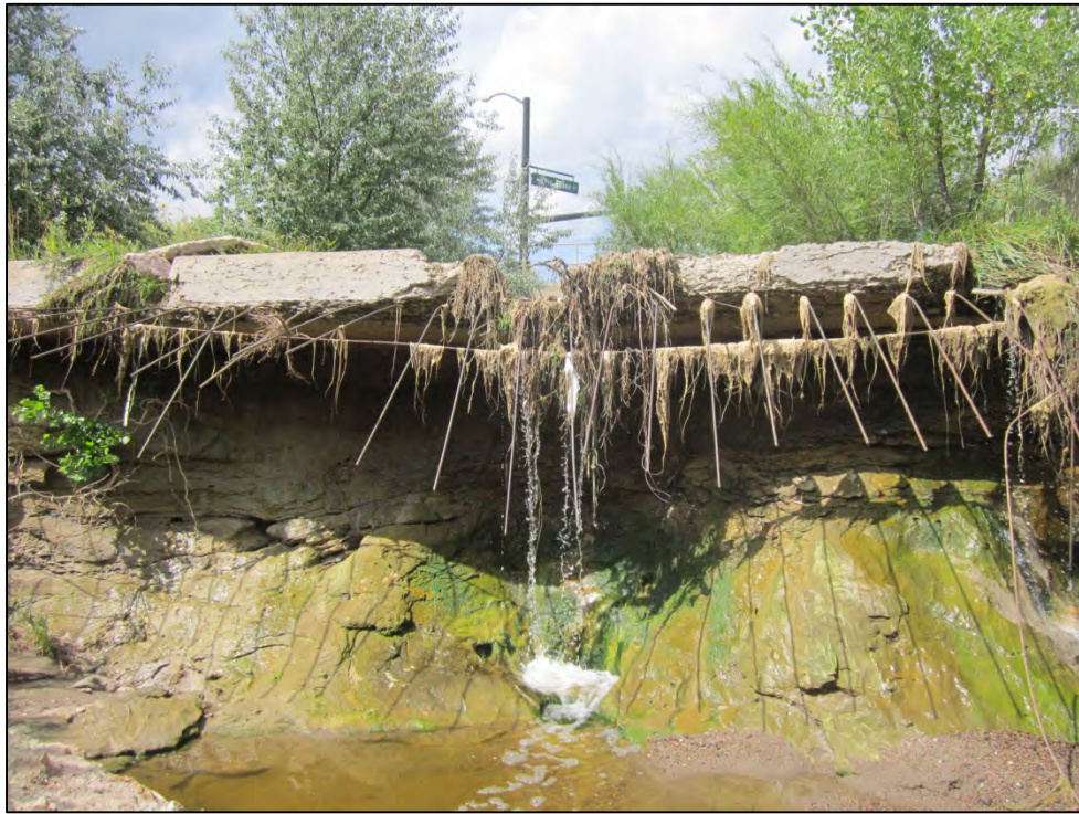
View, facing upstream, of unmaintained and deteriorated concrete drop structure in Rockrimmon Channel. Note the significant deterioration and undercutting of the concrete drop structure.
