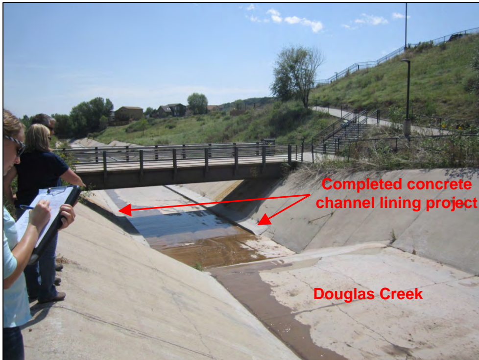
Photograph 16. View, facing downstream, of CS – 016 Location No. 1 completed concrete channel lining project on Douglas Creek near Intel Way.
