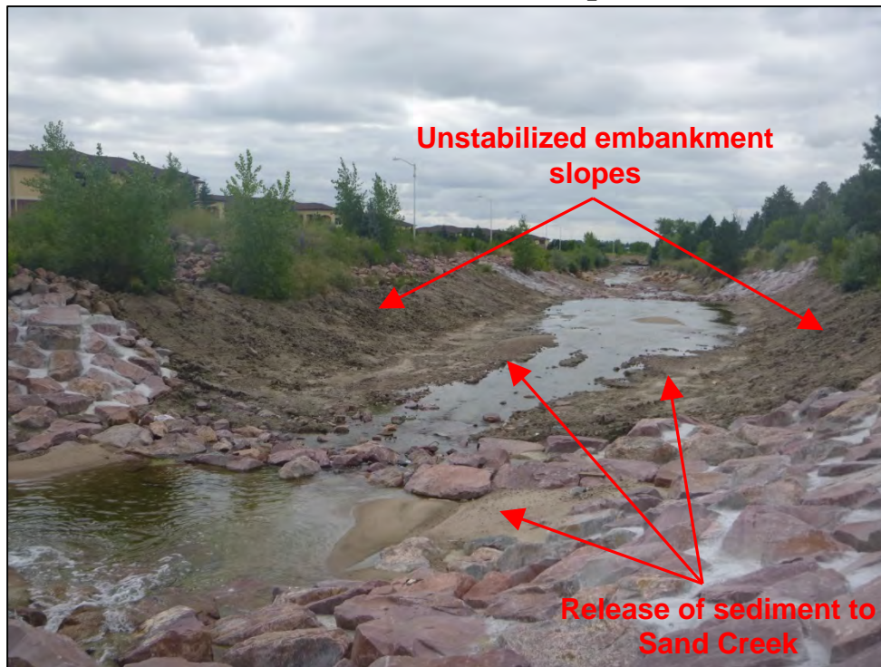
Photograph 93. View of unstabilized Sand Creek embankment slopes associated with the project and evidence of a previous release of sediment to Sand Creek.
