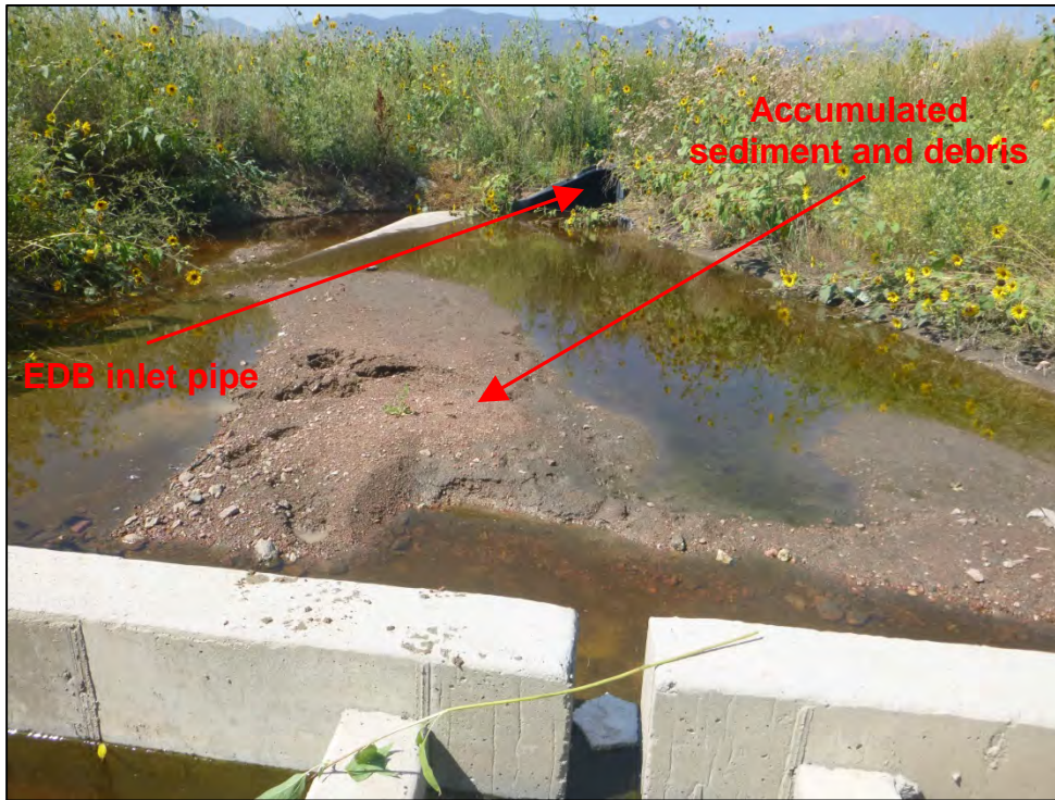
Photograph 11. View of ID-57 VA Hospital EDB inlet forebay with accumulated sediment and debris.
