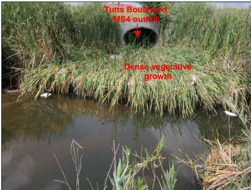
Photograph 123. View of unmaintained (e.g., dense vegetative growth) Tutts Boulevard MS4 outfall rip-rap flow dissipation device, which subsequently drains to Sand Creek Detention Basin No. 1.
