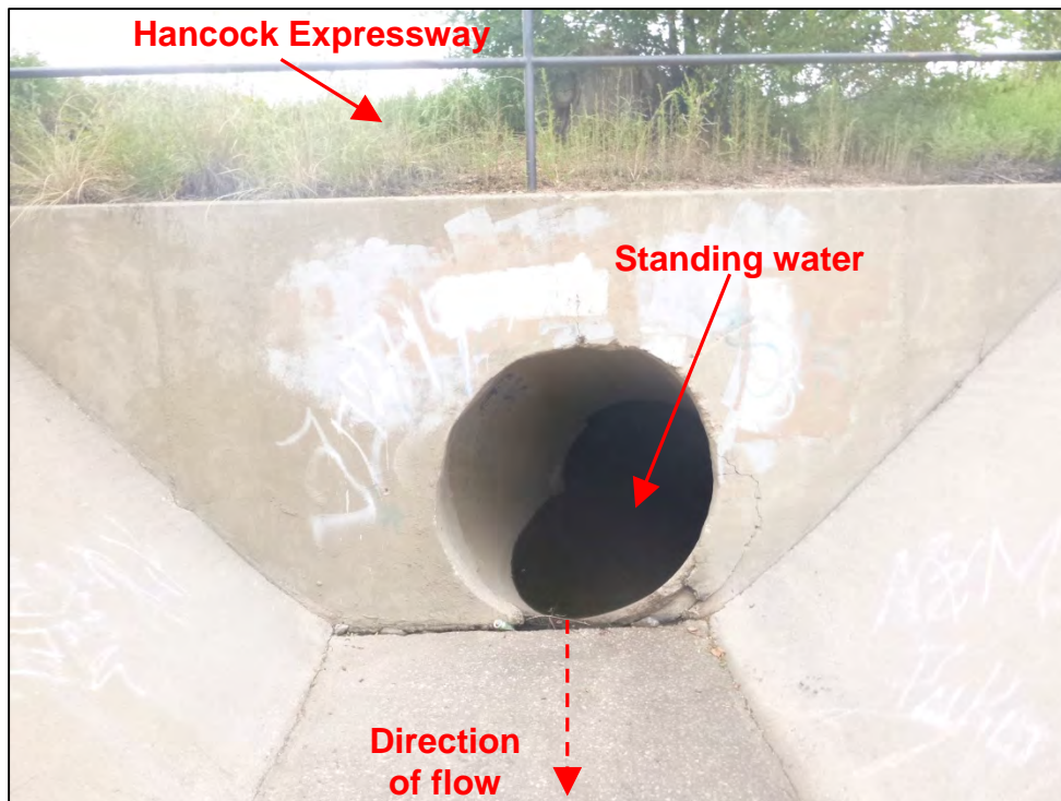
Photograph 64. View of CS – 060 Hancock Expressway Drainage culvert pipe outlet to concrete lined channel. Note the culvert pipe did not appear to be installed at the proper grade to convey flow as standing water was observed within the pipe.
