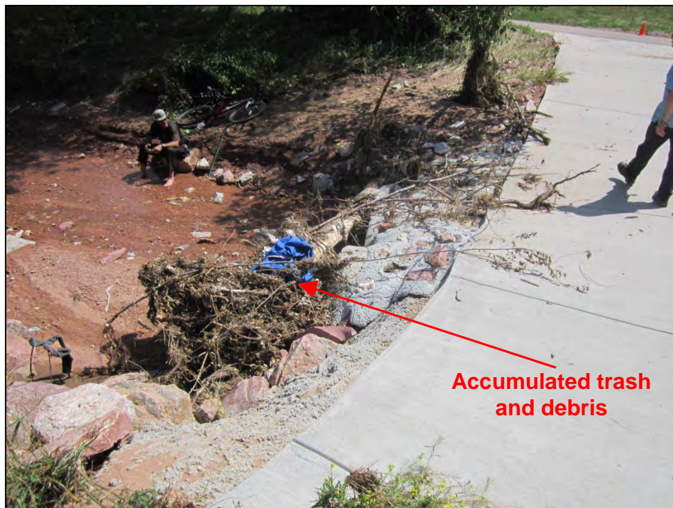
Photograph 20. Close-up view of accumulated trash and debris at culvert pipe inlets on the upstream side of the Douglas Creek low water crossing.
