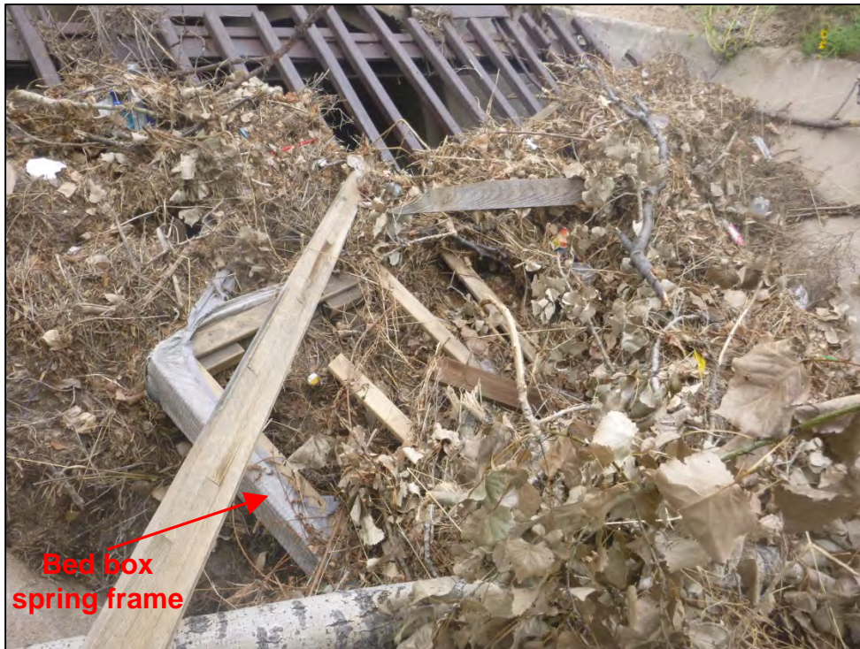
Photograph 69. Additional close-up view of trash and debris at the culvert pipe inlet trash rack. Note the bed box spring frame and other debris accumulation.
