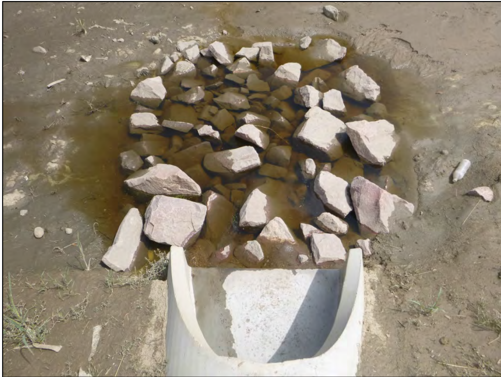
Photograph 127. Close-up view of accumulated sediment and debris at one of the three inlets and associated forebay.
