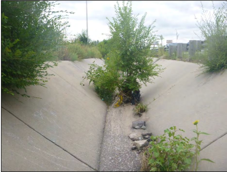
View of CS – 130 concrete lined MS4 conveyance channel. Close-up view of vegetative growth (e.g., shrubs) and accumulated debris in the channel.
