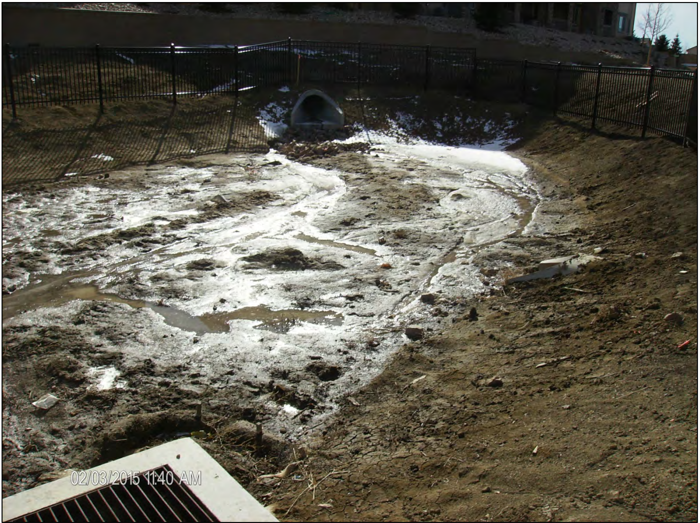
Exhibit 20. City provided photograph of ID – 070 Woodmen Ridge Apartments EDB, dated February 3, 2105. Note that the EDB was unstabilized and contained accumulated sediment and debris.
