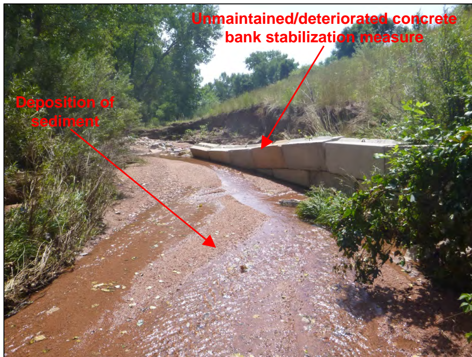
Photograph 22. View of an unmaintained and deteriorated concrete bank stabilization measure. Also note the deposition of sediment within Douglas Creek.
