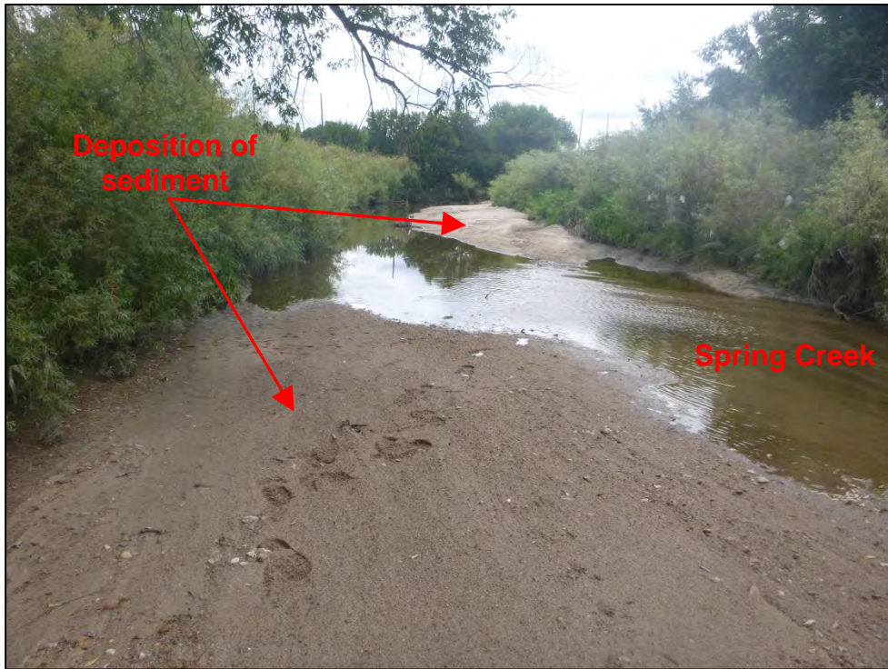
Photograph 87. View of significant deposition of sediment in Spring Creek located behind the private property residences on Teal Court.
