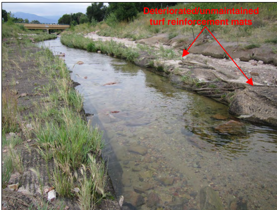
Photograph 104. View of BMPs (turf reinforcement mats) implemented in Sand Creek. Note the turf reinforcement mats were observed deteriorated and unmaintained.
