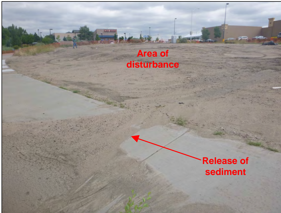
Photograph 99. Close-up view of a previous release of sediment across the sidewalk from the City contractor's unstabilized area of disturbance (i.e., staging area), shown in Photograph 97. Note the lack of erosion, sediment, and perimeter controls.
