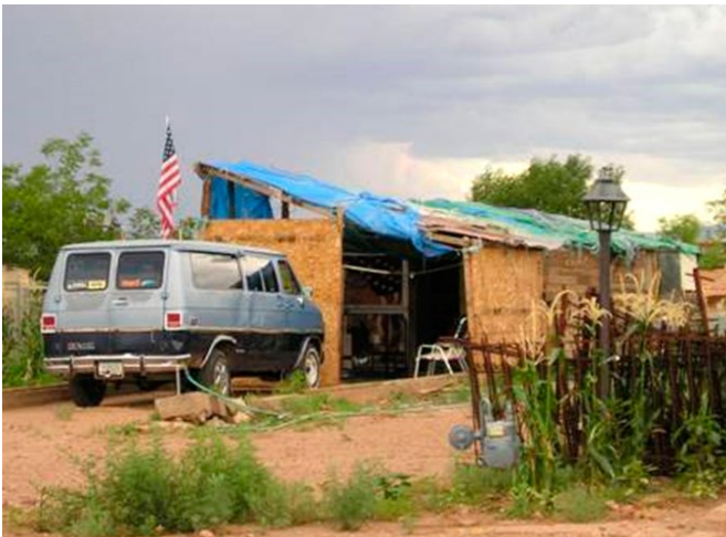
Many colonia homes are self-constructed from readily available used and new materials. Credit: EPA Office of Environmental Justice.
