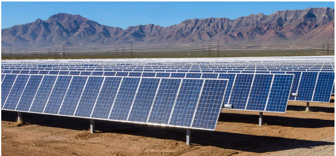
The Newman Solar, LLC facility in northeast El Paso, Texas, generates clean energy to power more than 3,800 homes. Credit: El Paso Electric.
