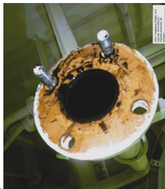
Oil residue in overboard discharge piping
