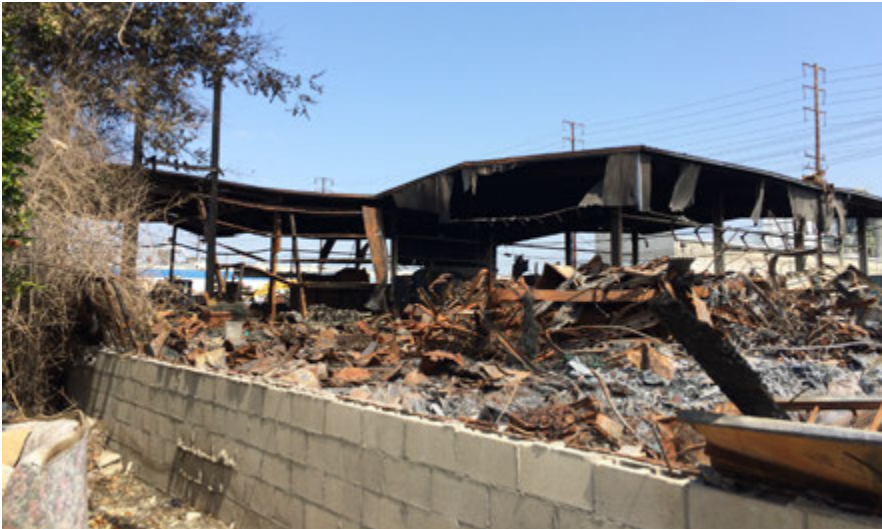
Debris to be removed by EPA at 3570 Fruitland Avenue
