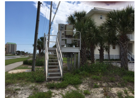
Elevate electrical panel
