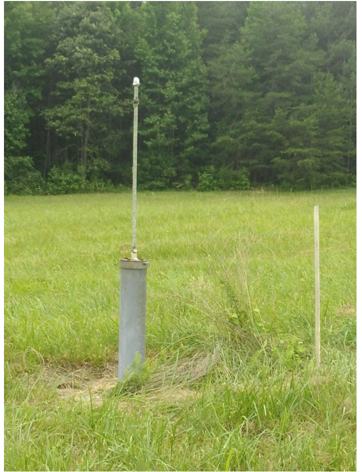
Picture 6: Wilcox Landfill – Passive Gas Vent
