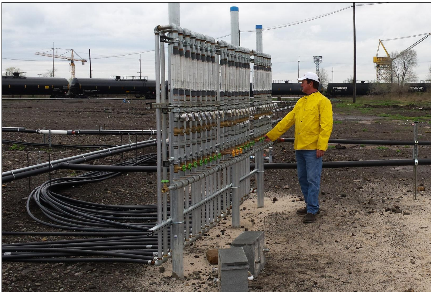
Cell 1 Upgraded Flow Control System
