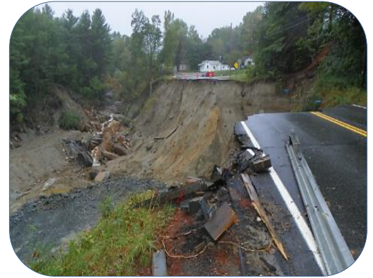
Upgrading transportation culverts will help Vermont prevent washed out roads and runoff into rivers and streams (seen above, after Hurricane Irene).
