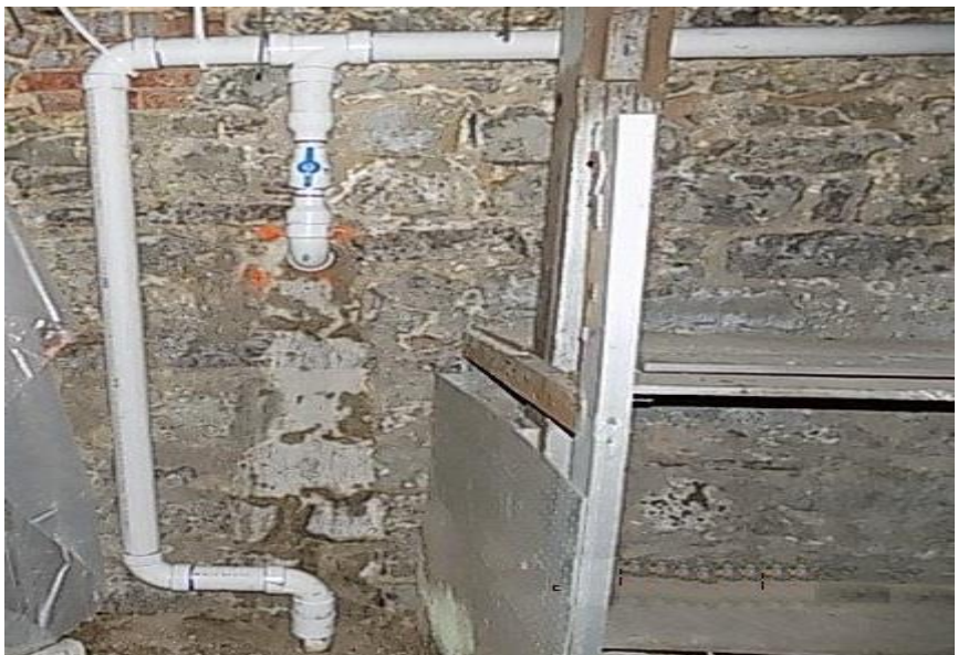
A section of the vapor mitigation system that helps prevent harmful vapors from entering basements.
