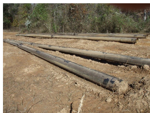
Asbestos Coated Pipeline
