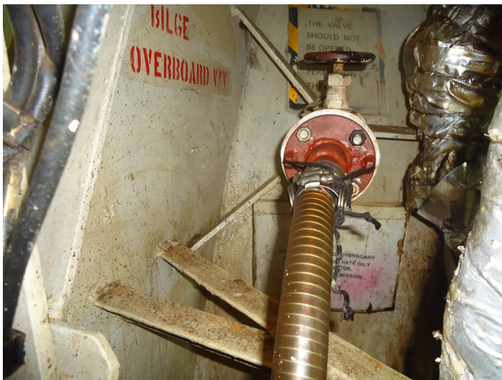
Bilge sent overboard with flexible hose.
