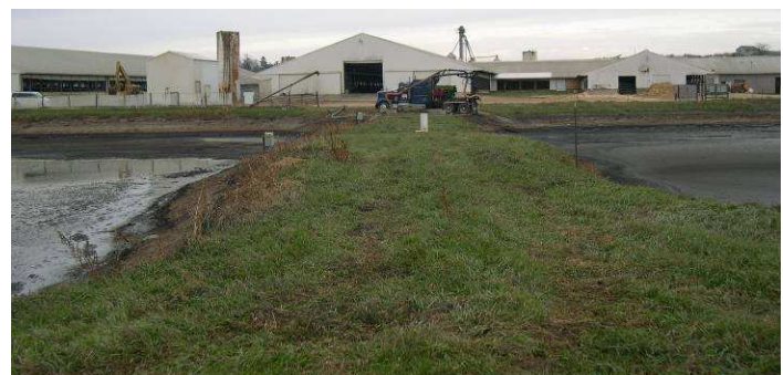
S side of lagoon looking E along the berm. 2 nd stage lagoon is on right.
