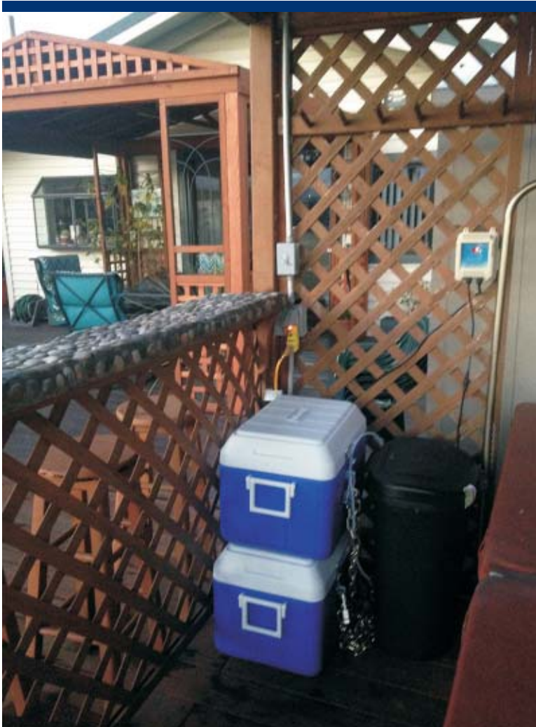
Photo 25 View of Viper Station JB01 at the Jantzen Beach Moorage Inc floating home community.
