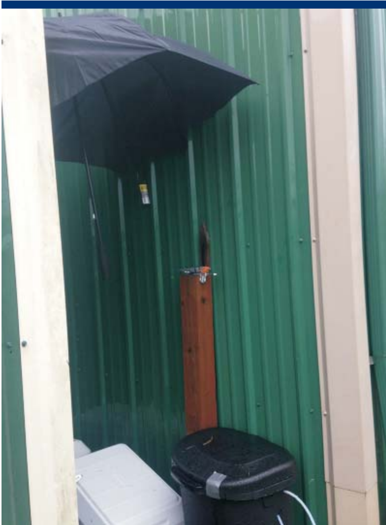
Photo 23 Umbrella used to protect Viper station while it is opened for maintenance. Direction: Southwest Date: 12/11/15 Time: 12:54
