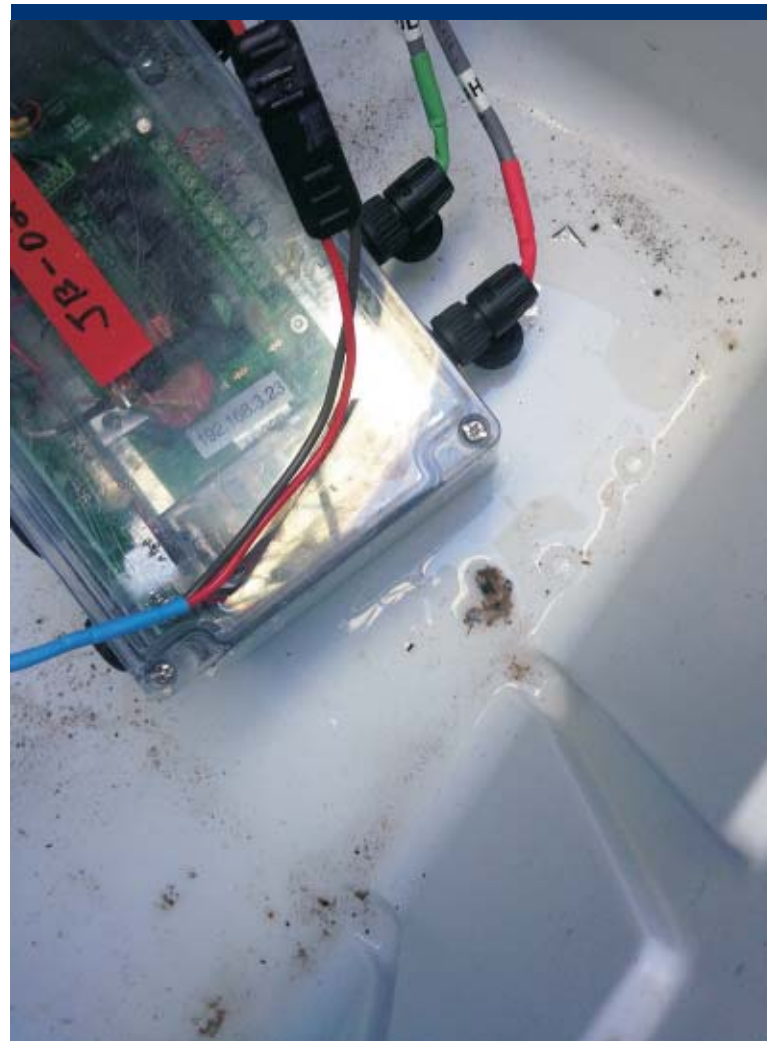
Photo 32 Viper station at JB02 is disassembled and water is visible in bottom of enclosure (not from leakage, but from condensation).
