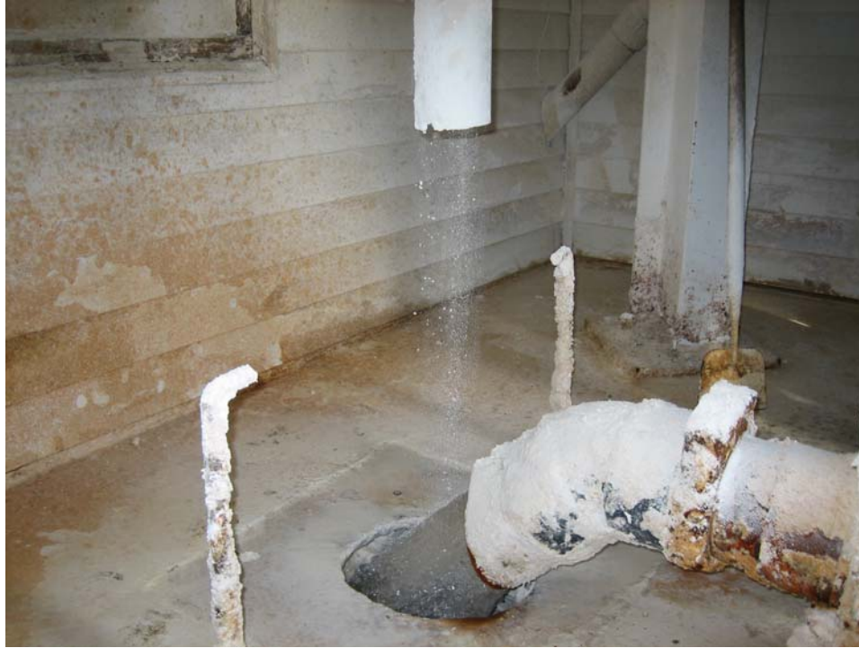
Figure 7-3. Photograph Inside the PBS Job #1 Lime House: AMD Flow and Lime Addition Source: Site Visit Report Pennsylvania Coal Mine Acid Drainage Treatment Systems (ERG, 2006)
