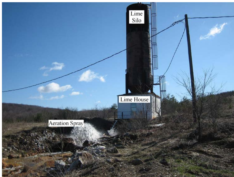
Figure 7-2. Photograph of the PBS Job #1 Lime House and Aeration Spray Source: Site Visit Report Pennsylvania Coal Mine Acid Drainage Treatment Systems (ERG, 2006)
