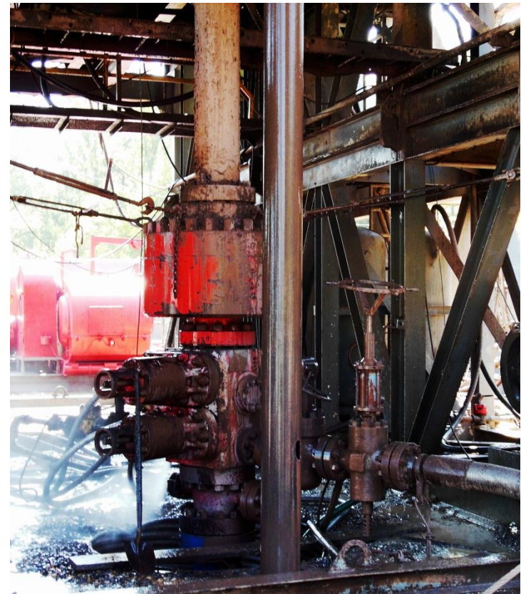
Wellhead Blowout Preventer
