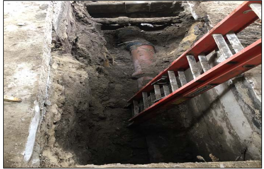
Photo 6: View facing south of clay sewer line with break in foreground
