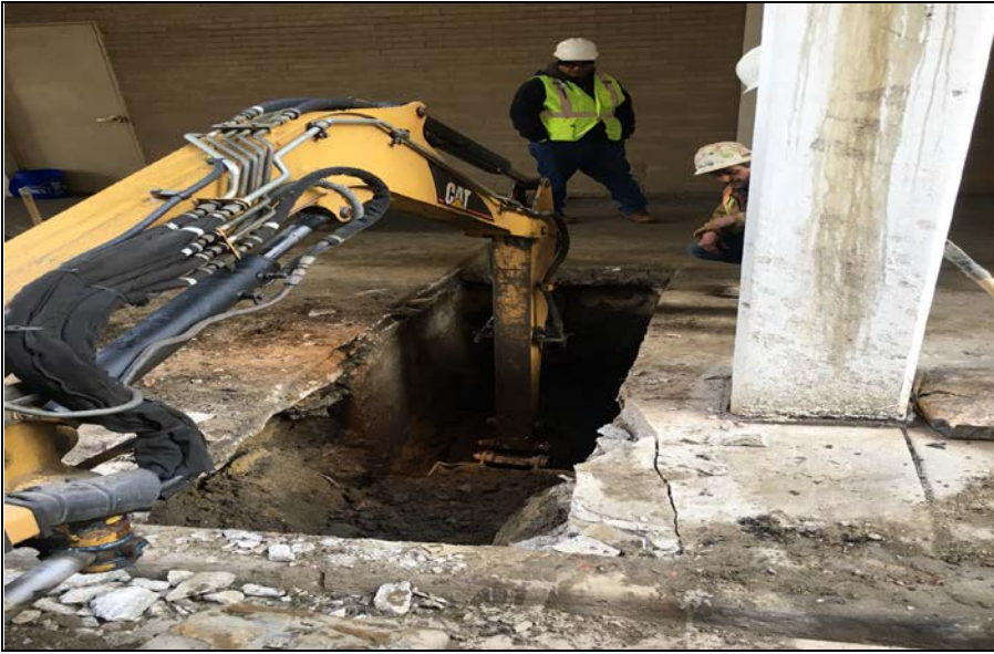
Photo 5: View facing north of excavating sidewalk for second break in sewer line
