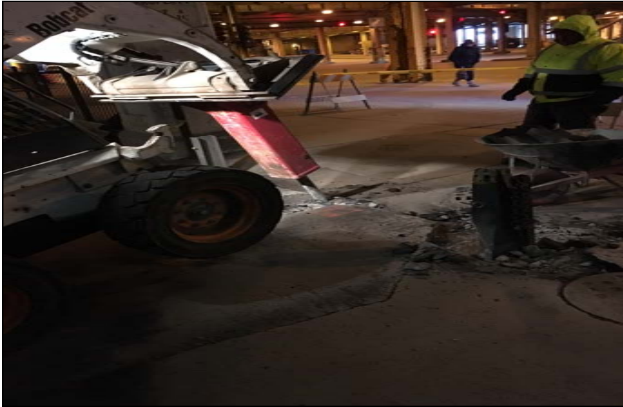
Photo 1: View facing southwest of Hole A concrete removal. Old rail in foreground to be removed.
