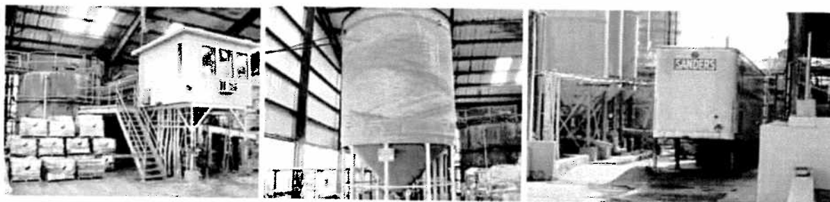
Figure 7. Settling tank & control room, sulfuric acid storage, trailer awaiting load of plastics.
