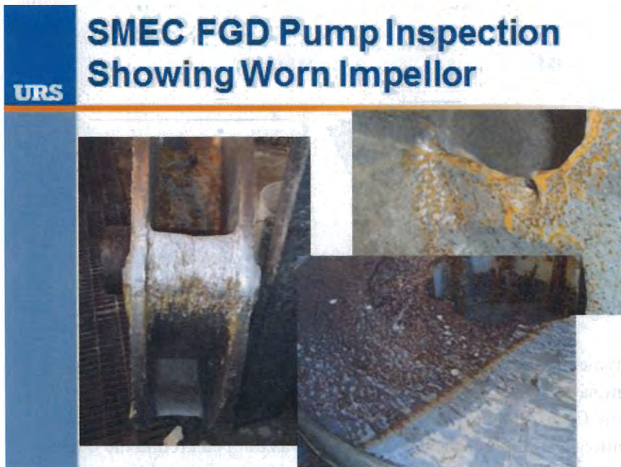
Figure 8.6. Inspection of San Miguel FGD Recycle Pump Showing Worn Impellor
