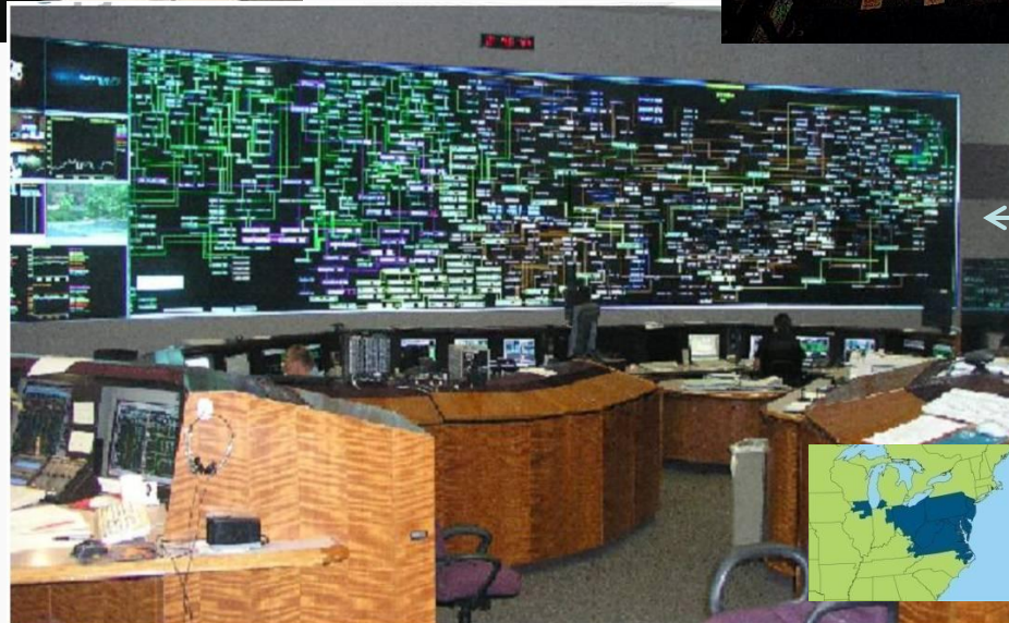
PJM's Control Room in Pennsylvania
