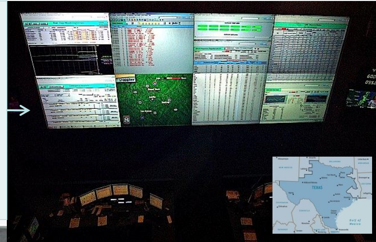
Electric Reliability Council of Texas (ERCOT) Control Room
