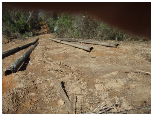
Asbestos Coated Pipeline
