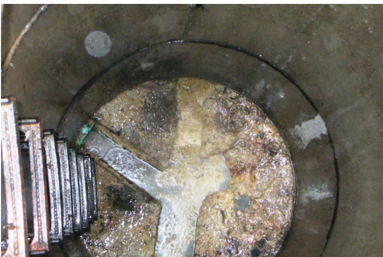
Southern Grease Pump Station
