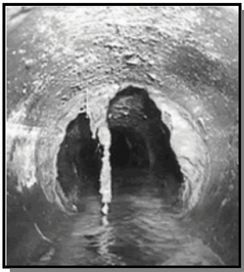
Root and grease buildup can cause blockages in a sewer system [photo: North Carolina Department of Natural Research (NCDNR)].
