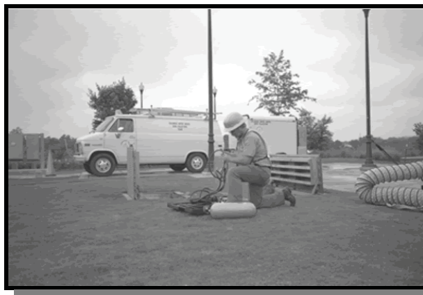
A sewer inspection is an important part of a sewer system capacity evaluation (photo: N.J. Department of Environmental Protection).
