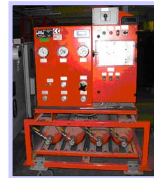
Dilo Model B120 5 Total Permanently Located @ Each Gas Insulated Gear Location
