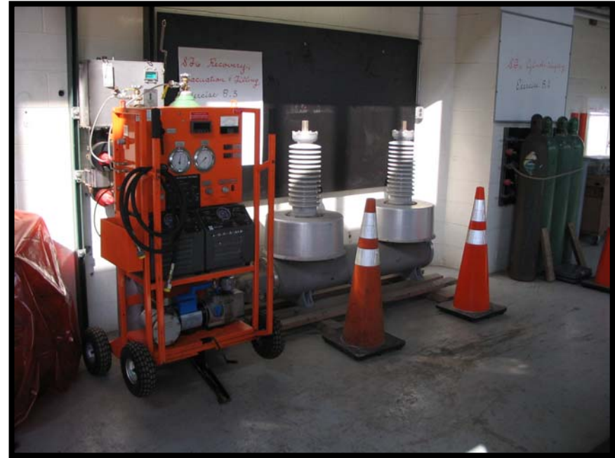
SF 6 Evacuation, Filling, and Recovery Hands-on Exercise (Shown Above)
