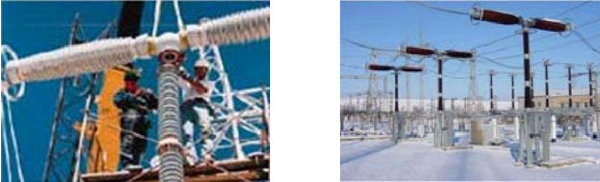
Figure 14. Typical old SF 6 puffer circuit breakers type live tanks to be maintained.
