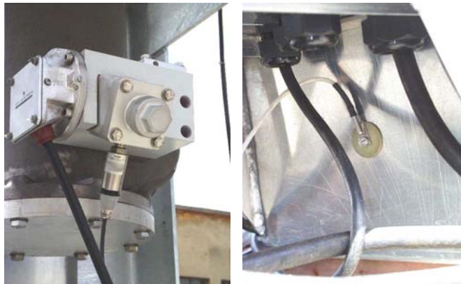
Figure 14. SF 6 pressure sensor and temperature probe
