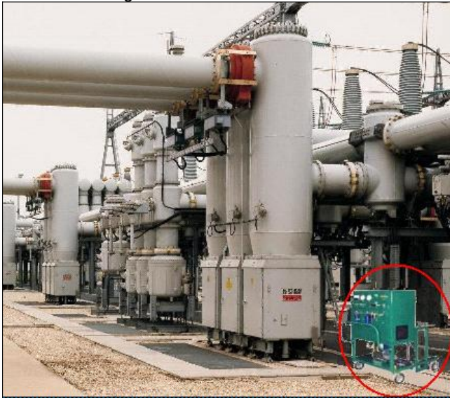
Fig. 10: Gas recovery unit.
