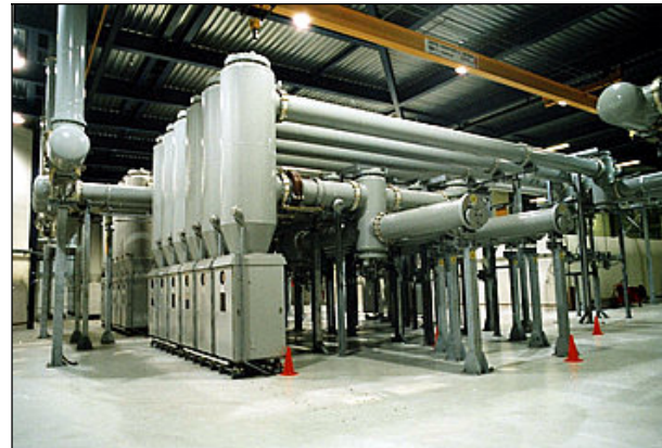
Fig. 2. Typical Gas Insulated Substation (GIS) 245 kV using SF 6 gas as insulation and interrupting medium. This is Gas Insulated Switchgear (GIS) as described later.
