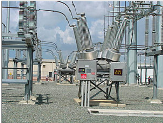
Fig. 3. Row of high-voltage circuit breakers with internal SF 6 gas insulation and connections to the bus air insulated with large energy losses on the buses.
