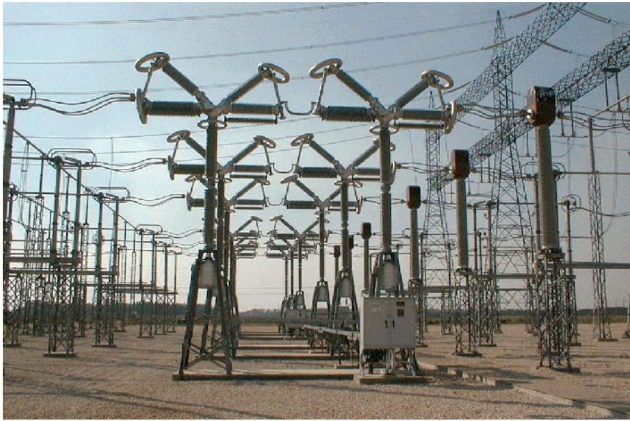
Picture 1: 500 kV SF 6 /CF 4 Live Tank Circuit Breaker at Manitoba Hydro's Dorsey Substation
