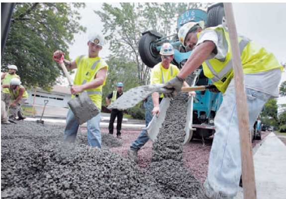
Crew installs a pervious concrete matrix in Shoreview, Minnesota (Photo by Bill Klotz).
